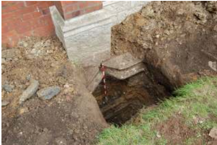
Fig 12 Oblique view of Test Pit 2 looking northeast and showing the large masonry blocks uncovered in the watching brief.
