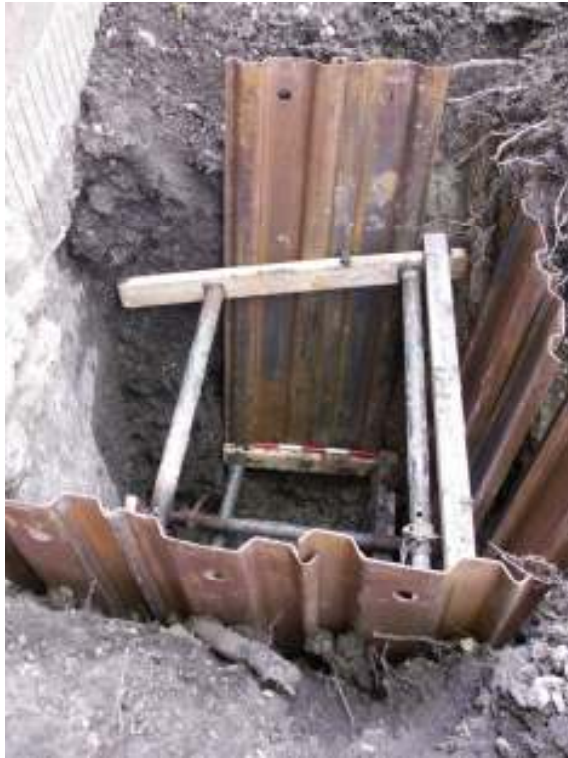
Fig 19 Test Pit 4 looking west and showing made ground deposits after machine extension.
