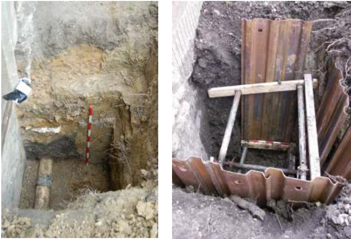
Fig 15 Test Pit 3, looking north. Right: the initial hand excavation TP and left the second phase after machine excavation. The same large fragment of polystyrene can be seen to the left of both images in the construction cut for the service pipe/construction of the Store building.
