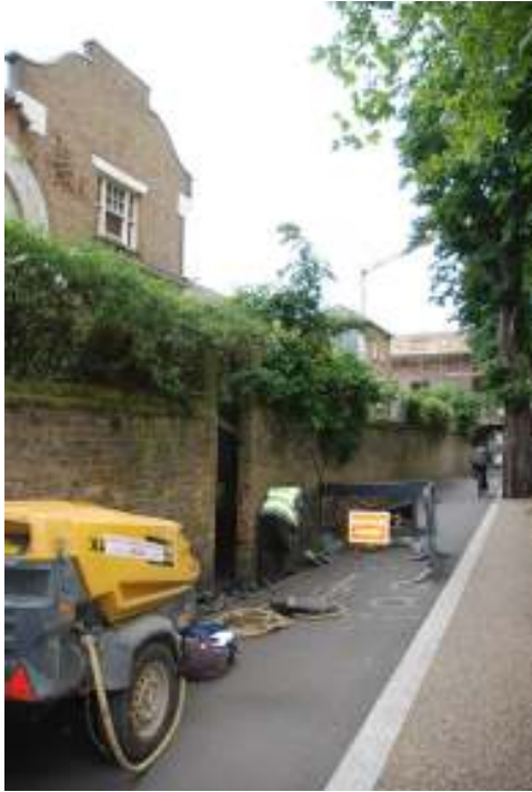
Figure 4 Location of the southern trench on Churchwell Path looking approximately south, the Dutch gable end of No. 27 Sutton Square can be seen.
