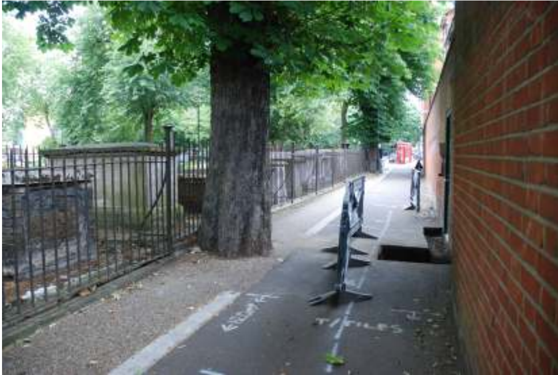
Figure 2 Location of the northern trench on Churchwell Path, looking north, the entrance gate to the Police Station can be seen to the right of the gully excavation, the soakaway is in the foreground.
