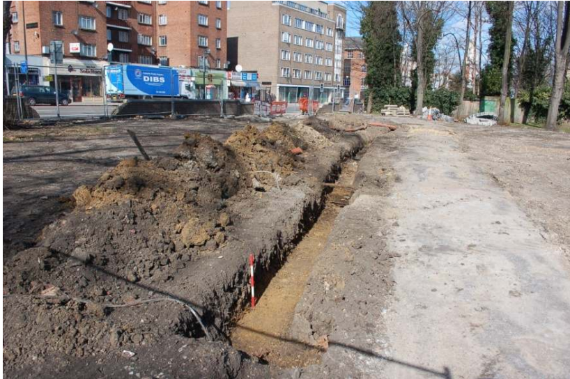
Figure 18: Pipe trench in Area A, view north towards Brixton Hill (0.5m scale).
