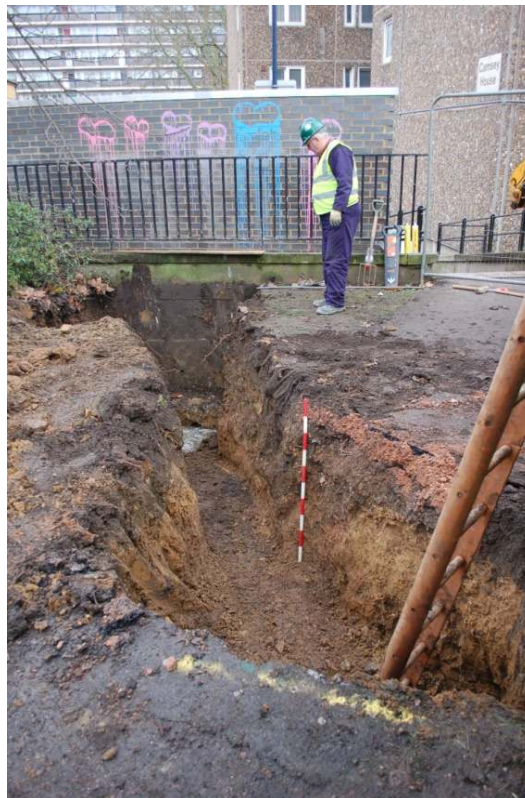
Figure 20: Connection trenching between the control kiosk and drive shaft outside the site compound (1m scale).
