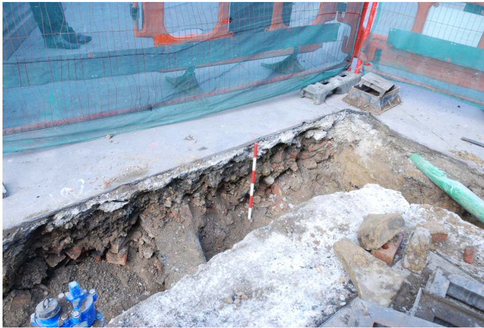
Fig. 35: View of one of the trenches at the northern end of Jewry Street (service backfills)
