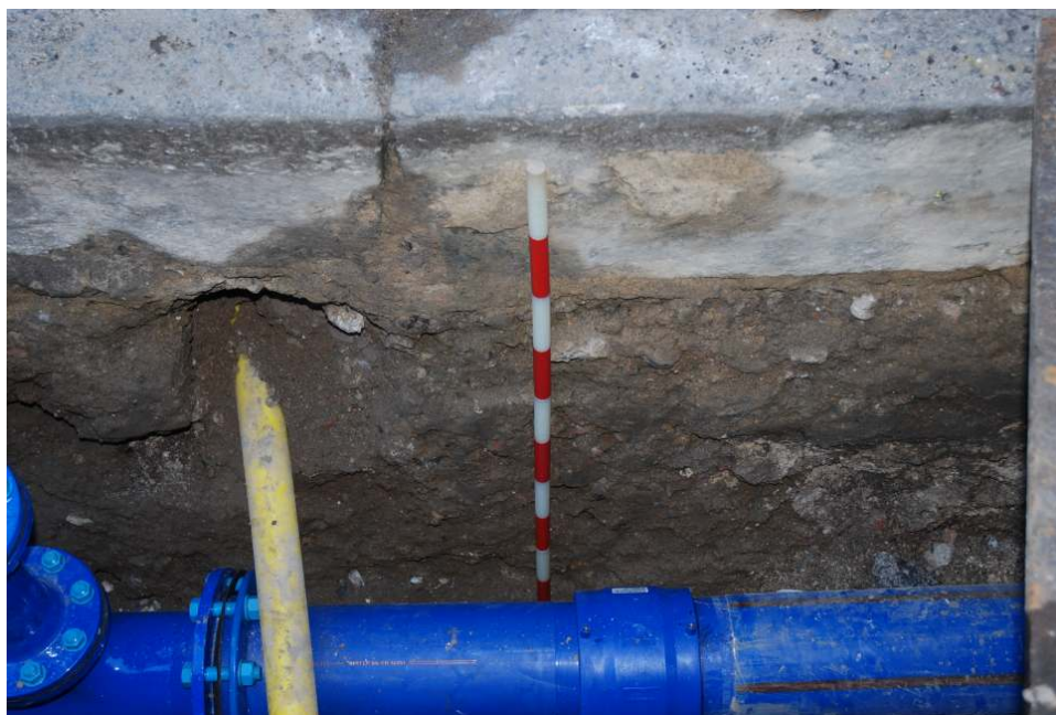
Fig. 37: View of India Street trench (disturbed by previous services and solid concrete base)
