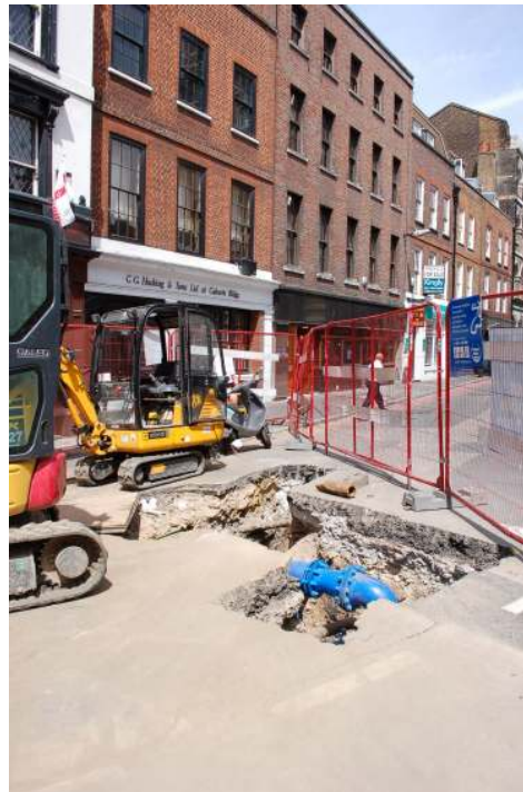
Figure 12: Trenching on the western fork of Borough High Street in the vicinity of Calverts Buildings, June 2010 ( cf. Fig 8 top left image).
