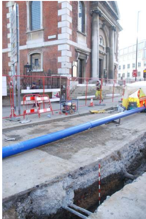
Figure 24: Trenching in the area of St George the Martyr's Church, Borough High Street ( cf. Cover and frontispiece).
