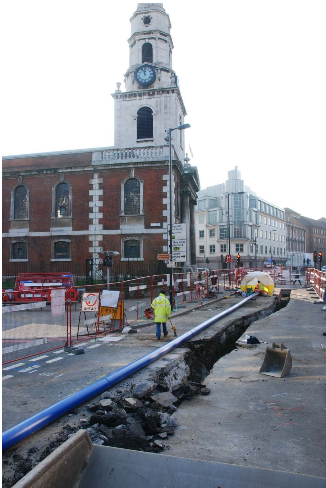
Frontispiece: General view of mains replacement works outside St George's Church looking south at the junction of Tabard Street.
