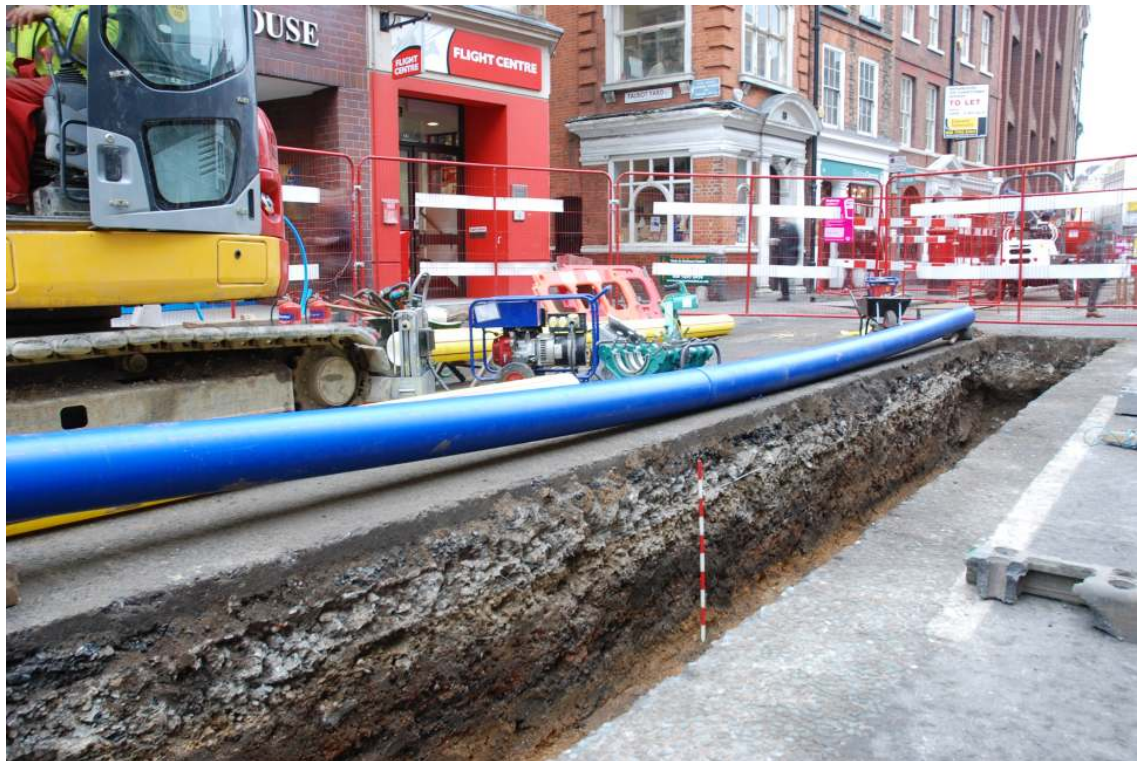
Figure 10: Top Right Trenching outside Nos 91-95 looking northeast, interestingly here the earlier road makeup layers survived as just a 20 to 30mm thick slither of in situ deposits, cut to the east and west by large later service trenches. The brown and yellow deposits (visible by the scale, top right) peel off to reveal the modern green sand service fills immediately behind. Below and Top Left: Slightly further south showing the west facing section of trenching between George Yard and Talbot Yard, looking south below and northeast above (19/01/10).
