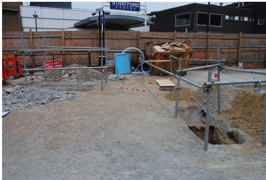
Figure 6: Locations of trial pits outside the Stratford Centre (July 2010). Trial pit A is to the left of the scale, Test pit B is just to the right of the scale (by the wooden board) and Test pit C is in the foreground to the right of the image.
