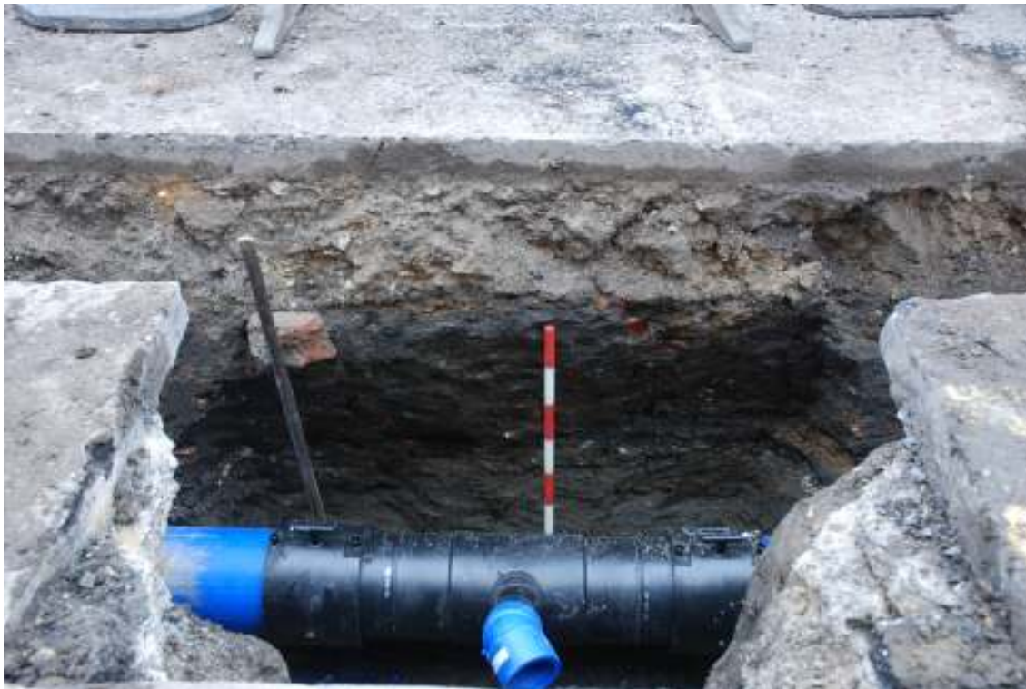
Fig. 34: Photo showing black 'surface' layer, trench 25, Paradise Street (running approximately midway across the scale)
