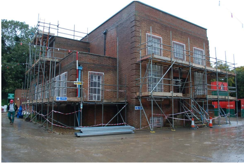
Figure 4: Matt's Hill Pumping Station from the main entrance on Cox Street Road.
