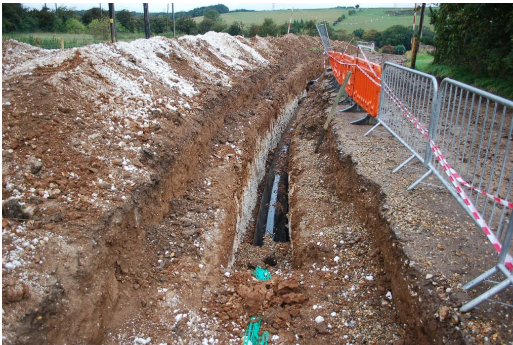
Figure 13: East end of open pipe trench in Field 2 showing rising chalk deposits.
