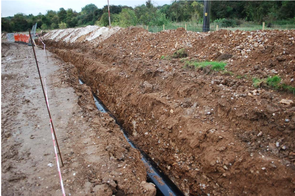
Figure 12: West end of open pipe trench in Field 2 showing clay and flint drift deposits, as can be seen it was difficult to enter the trenches at all locations owing to Health and Safety constraints.
