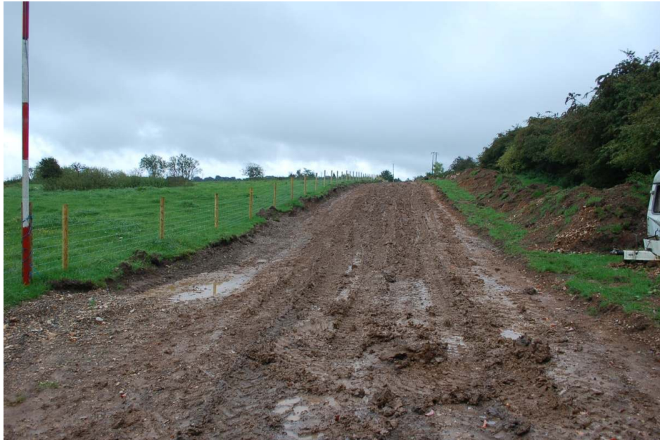
Figure 5: Field 1 from the gated entrance on Cox Street Road, looking southeast along the route of pipeline and easement corridor.
