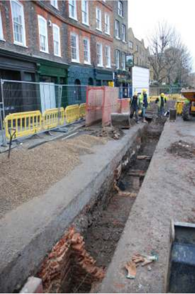
Fig. 49: Photo looking west along trench, showing context [41] in the foreground, and context [46] in the background, with fill [45] between them
