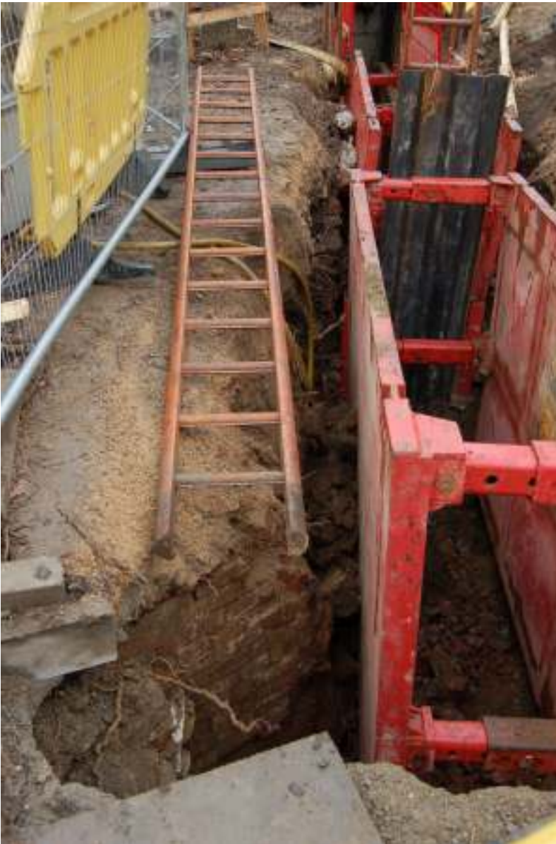
Fig. 14: Photo of basement wall (left foreground below the ladder), in the northern part of the trench running from the northern edge of Narrow Street across the open park
