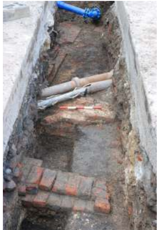
Fig. 63: Photo of section 12, looking west, with context [63] (underneath the scale), and context [67] beyond (forming the outline of the building)
