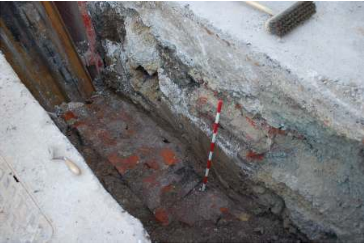
Fig. 30: Photo of context [9] (brick wall), with contexts [12] and [13] (chalk and alluvial clay) to the south of this, looking south
