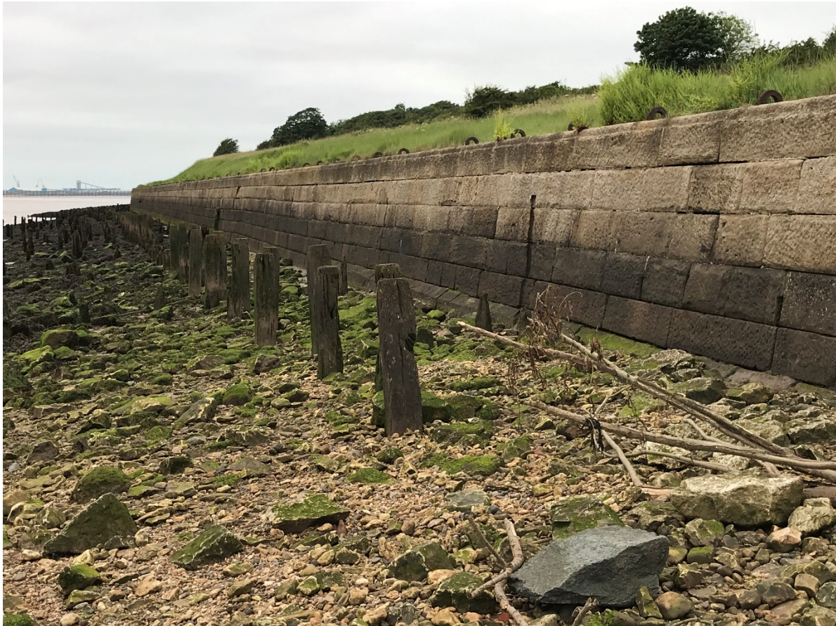
Figure 11.1 Paull Point Coastal Battery – in places it is at risk of coastal erosion.
