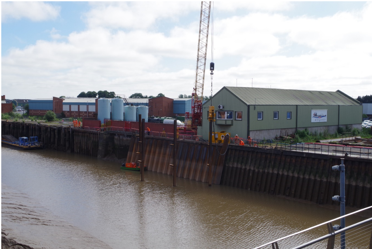
Figure 10.2 Flood defence improvements on the River Hull at Citadel Wharf, Hull in 2019.
