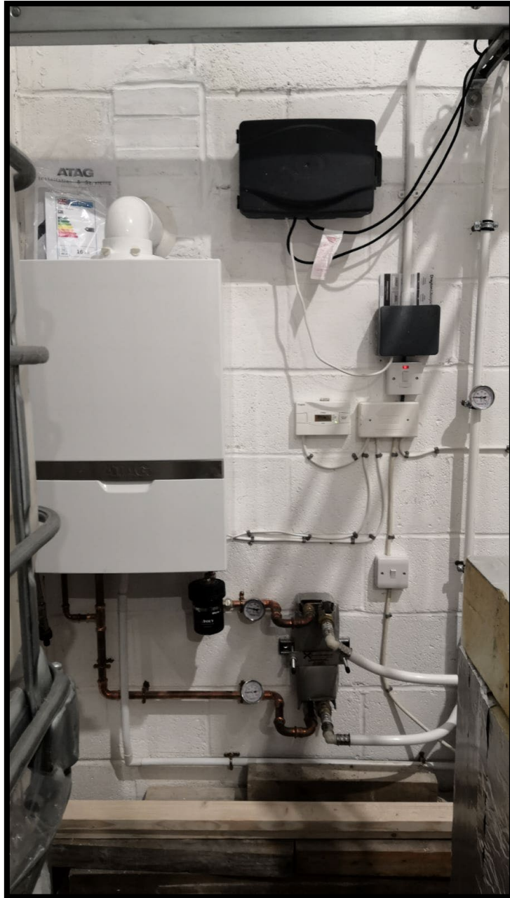
Figure 6; The gas heating system heating the PEG inside the tank.
