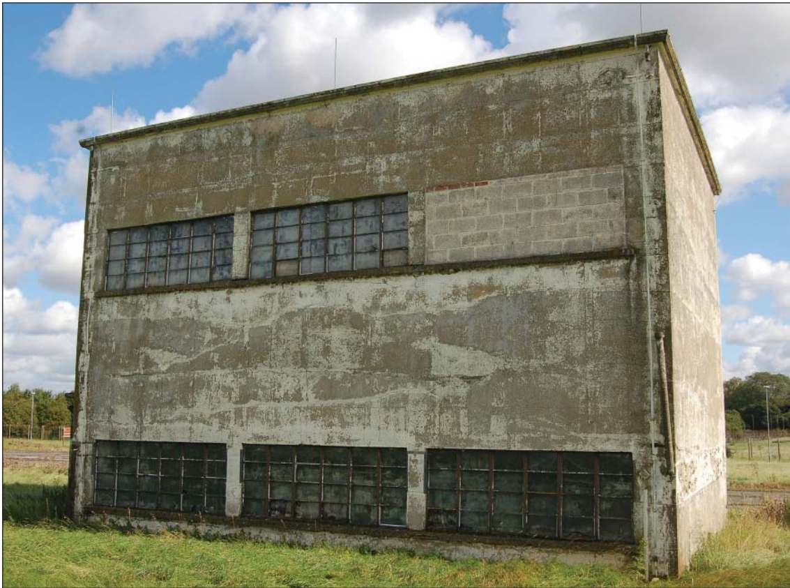
Figure 8: RAF Upper Heyford, rear view of the early 1950s Strategic Air Command 'A' Structure, the capsule or trigger store (1007) , similar designs are found in continental USA. It is claimed that these buildings exhibited a remarkable similarity with the first SAC headquarters building at Offutt, Nebraska, designed by Albert Kahn for the Martin Bomber Plant. (c) C. Welch
