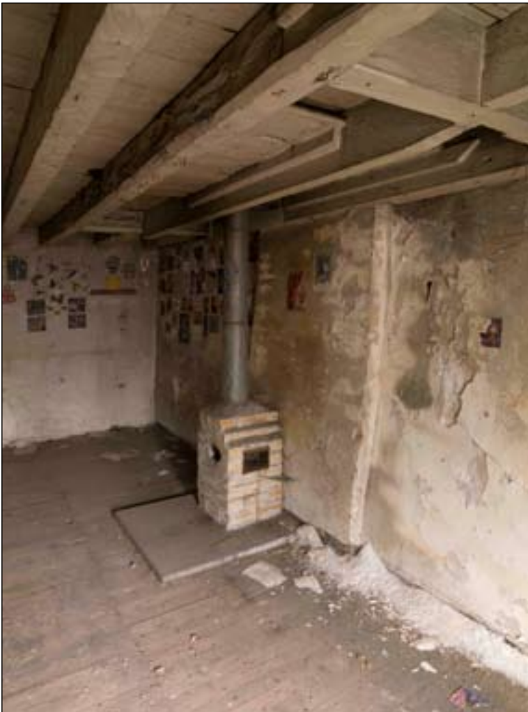
Fig. 47: Evidence for the stair position on the second floor of the granary. DP065359 © English Heritage
