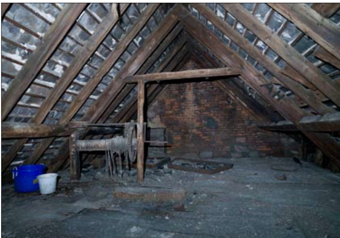
Fig. 74: The roof of the main range of 57 West Street / 64-66 Bridge Street, looking west. The winch is associated with a low loading doorway in the gable beyond. DP065403 © English Heritage
