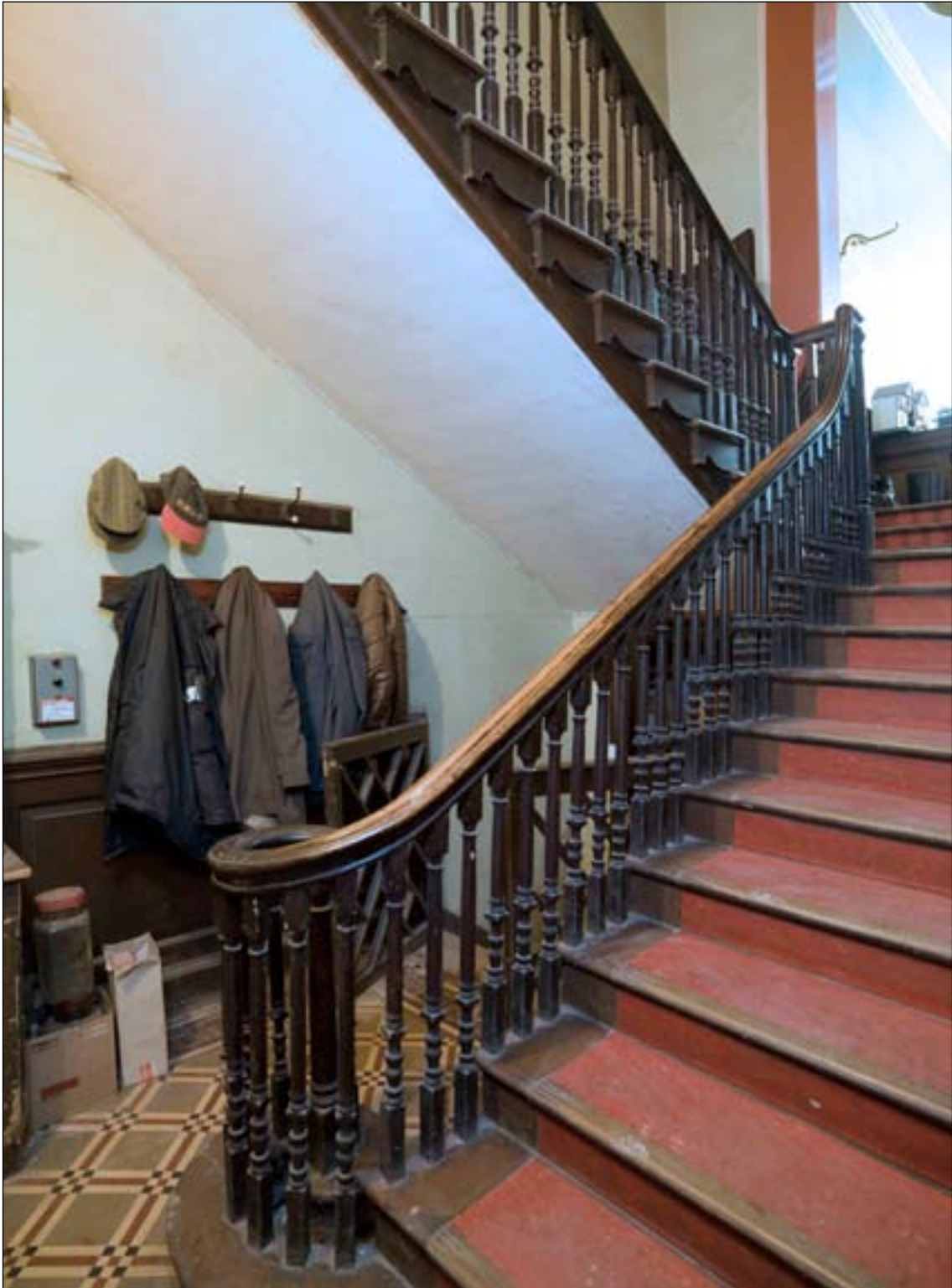
Fig. 17: The principal staircase of 2 Love Lane / 64 West Street with curtail, ramped handrail and three column balusters per step. DP065331 © English Heritage
