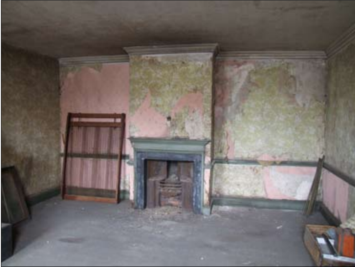
Fig. 26: The larger second-floor bedroom with stone chimneypiece, 2 Love Lane / 64 West Street. © English Heritage
