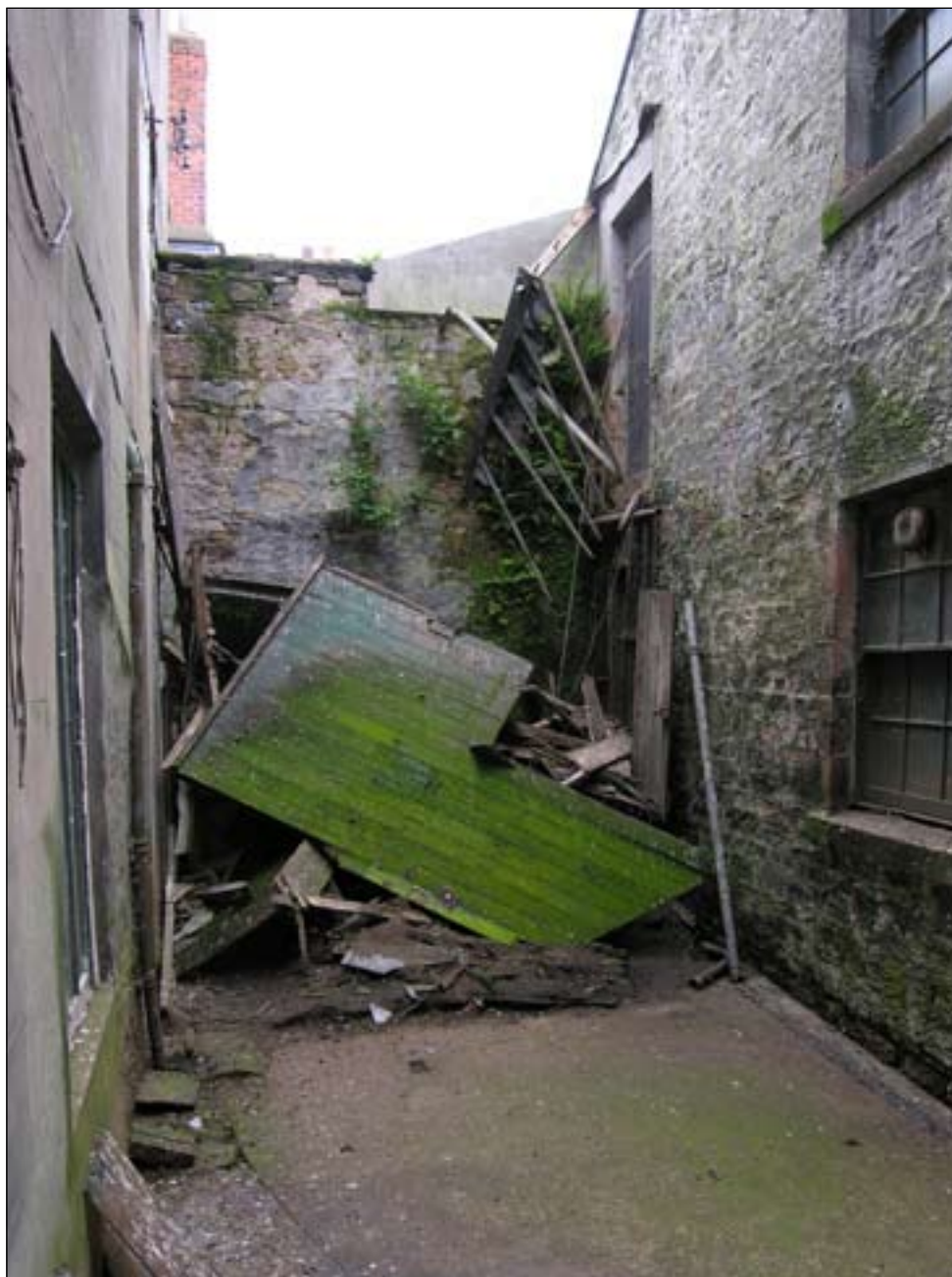
Fig. 53: The collapsed timber corridor which crossed the internal yard between 2 Love Lane / 64 West Street and the granary (60 West Street). © English Heritage
