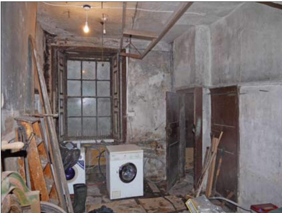
Fig. 20: The original kitchen of 2 Love Lane / 64 West Street., looking east towards the 'inside yard'. The two doorways to the right relate to originally separate lobbies, one opening off the 'inside yard', the other leading to the dining room and stair. © English Heritage
