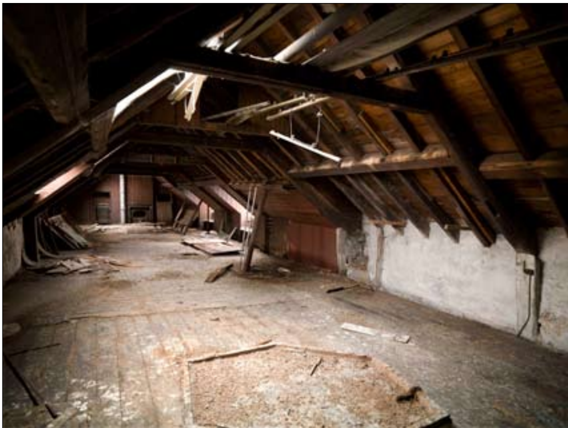
Fig. 48: View of the attic of the granary, showing the collar trusses, looking east, with John Wilson's late 19th-century office at the far end. DP065356 © English Heritage
