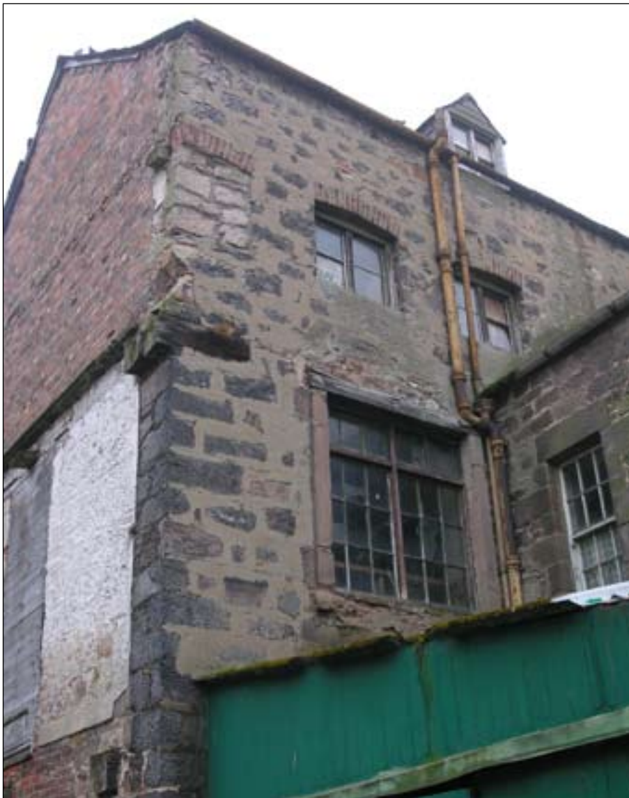
Fig. 43: First floor window with stone surround in the southern wall of the granary west of the outshot. © English Heritage
