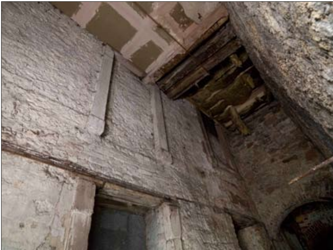
Fig. 40: View of the covered ground-floor passage extending along the north side of the granary, showing original openings (with raised surrounds) in the north wall of what was once the coach house and stables. DP065314 © English Heritage
