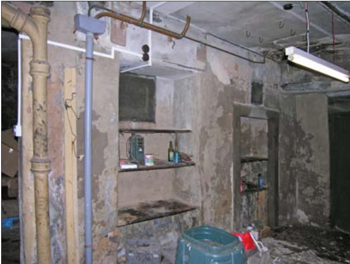
Fig. 42 (below): Blocked ground-floor openings in the southern wall of the granary. © English Heritage
