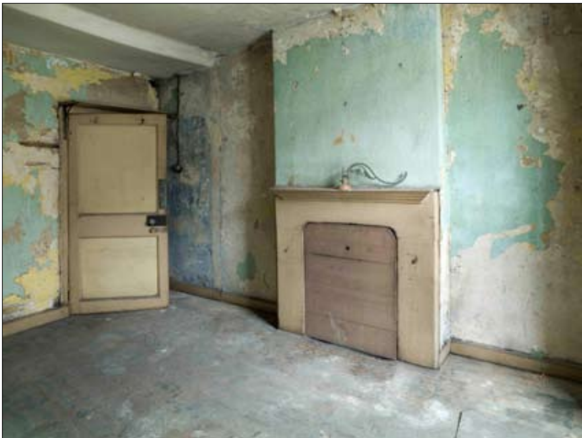
Fig. 71: The bedroom on the western end of the second floor of the outshot, 57 West Street / 64-66 Bridge Street. DP065393 © English Heritage
