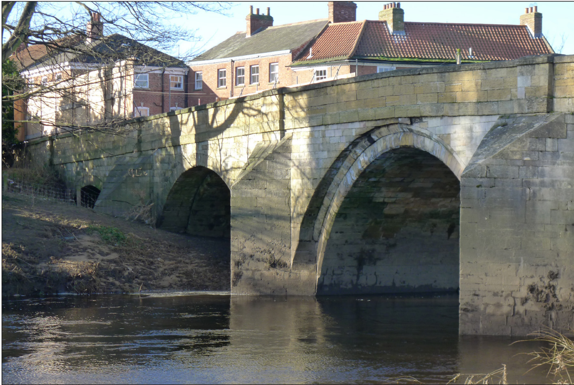
Figure 7: View of the squinch arch springing from the crown of arch 5 on the downstream side of the bridge. Note the difference in the form of the arch rings: the extension associated with the squinch arch has effectively refaced the western spandrel of arch 5 and all subsequent arches in the western half of the bridge. Note also the difference in the colour of the parapet's stonework. (AF00398018 © Historic England/Lucy Jessop).
