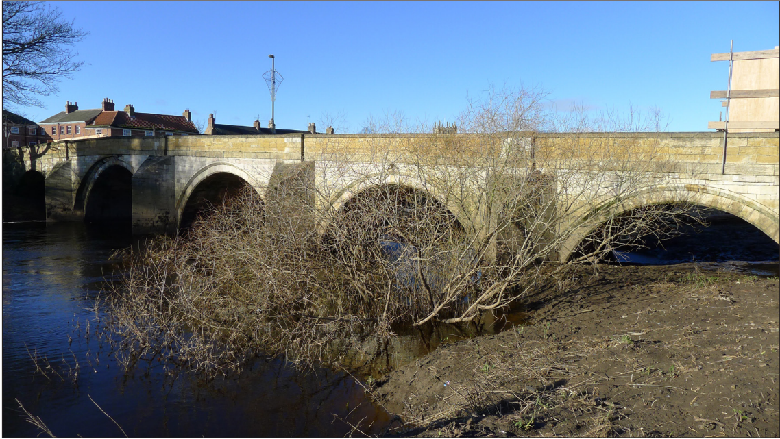
Figure 3: The downstream arches 2 to 5 (from right to left) of the 1698 bridge, showing the problems of silting in arch 2. (AF00398015 © Historic England/Lucy Jessop).
