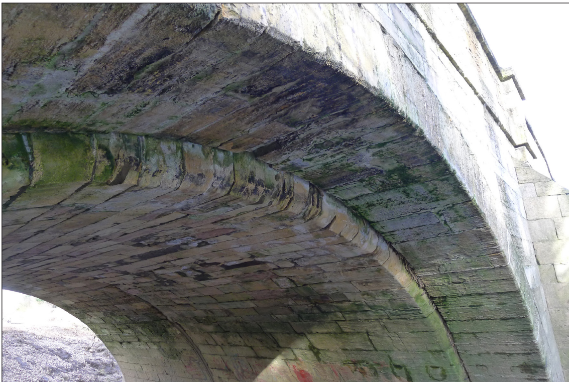
Figure 8: The intrados of arch 6, showing the 1698 bridge (centre) flanked by the new arches for (right) the downstream extension and (left) the 1791 upstream widening. (AF00398057 © Historic England/Lucy Jessop).
