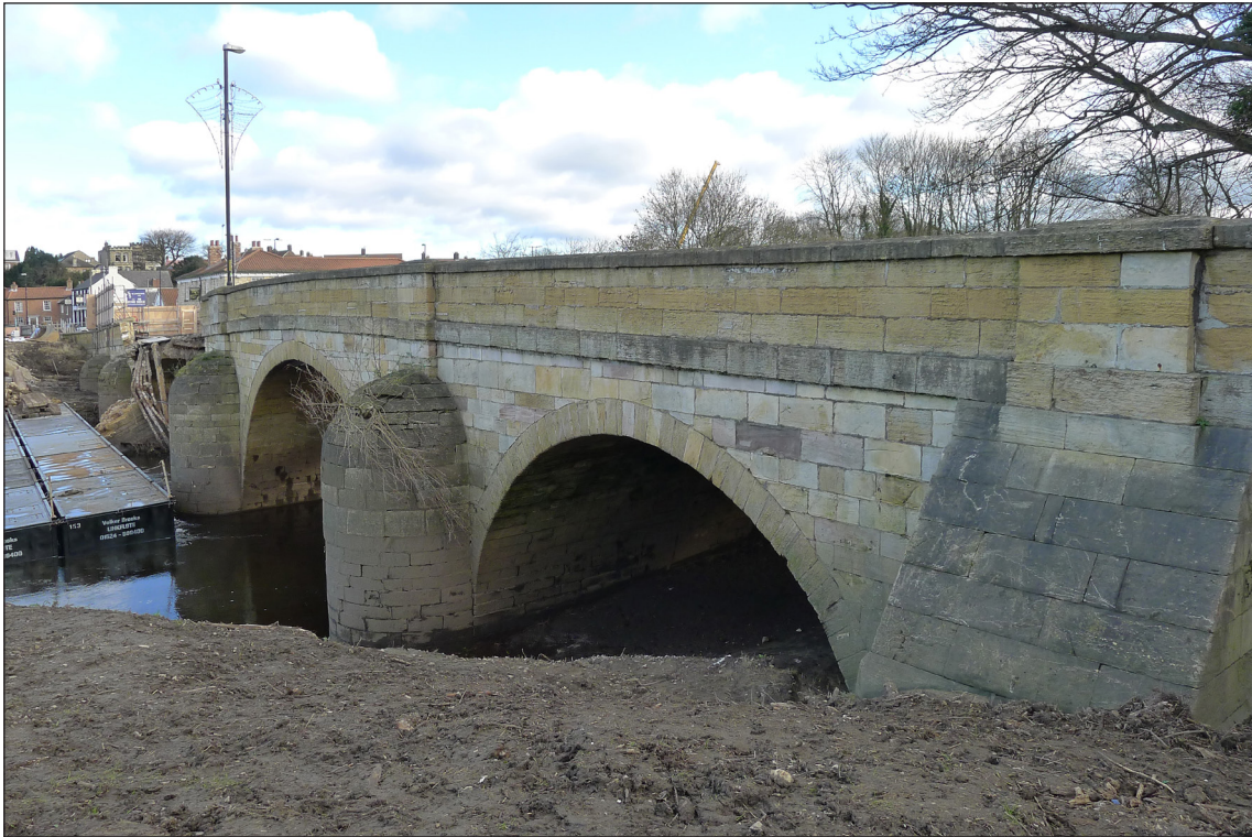
Figure 9: The 1791 upstream widening, with its vast, cylindrical, bull-nosed cutwaters. Note the different form of the cutwater against pier 6 (right of frame). (AF00398046 © Historic England/Lucy Jessop).
