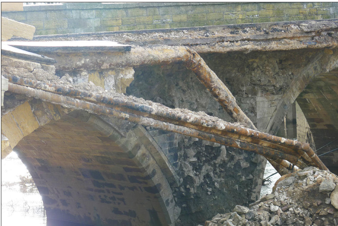
Figure 10: View of the collapsed (upstream) pier 3 of the 1791 bridge. Note the arch ring, archivolt, spandrel-facing and exposed scar of the removed cutwater of the exposed 1698 bridge behind, with arches 3 and 4 all apparently undamaged. (AF00398043 © Historic England/Lucy Jessop).
