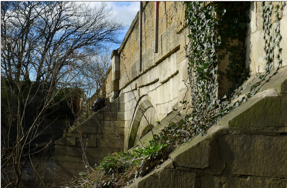
Figure 6: View westwards along the downstream elevation of arch 2. The oversailing course of ashlar immediately above the archivolt is not displaced or bulging stonework, but the remains of the original string course superseded by a new, higher, string course when the deck was raised and flattened out. (AF00398024 © Historic England/Lucy Jessop).
