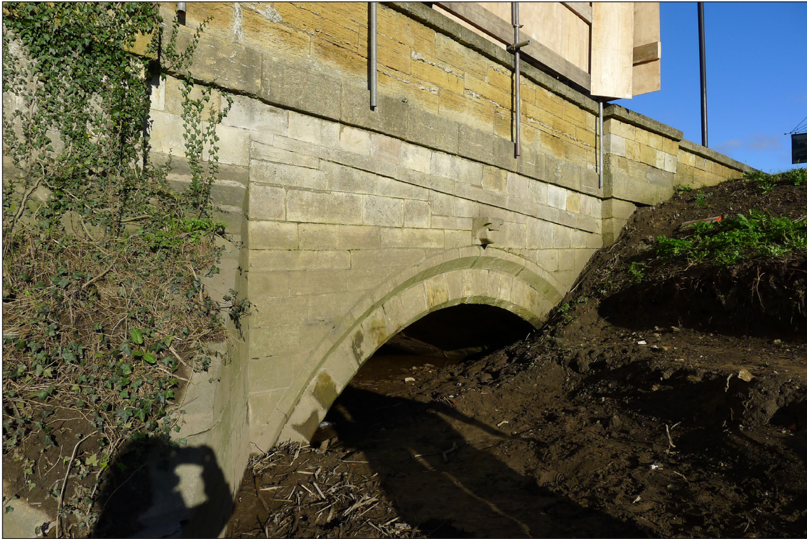
Figure 5: The downstream elevation of arch 1, showing the string course and lowest course of the parapet as built in 1698 surviving below the present heightened deck level. (AF00398011 © Historic England/Lucy Jessop).
