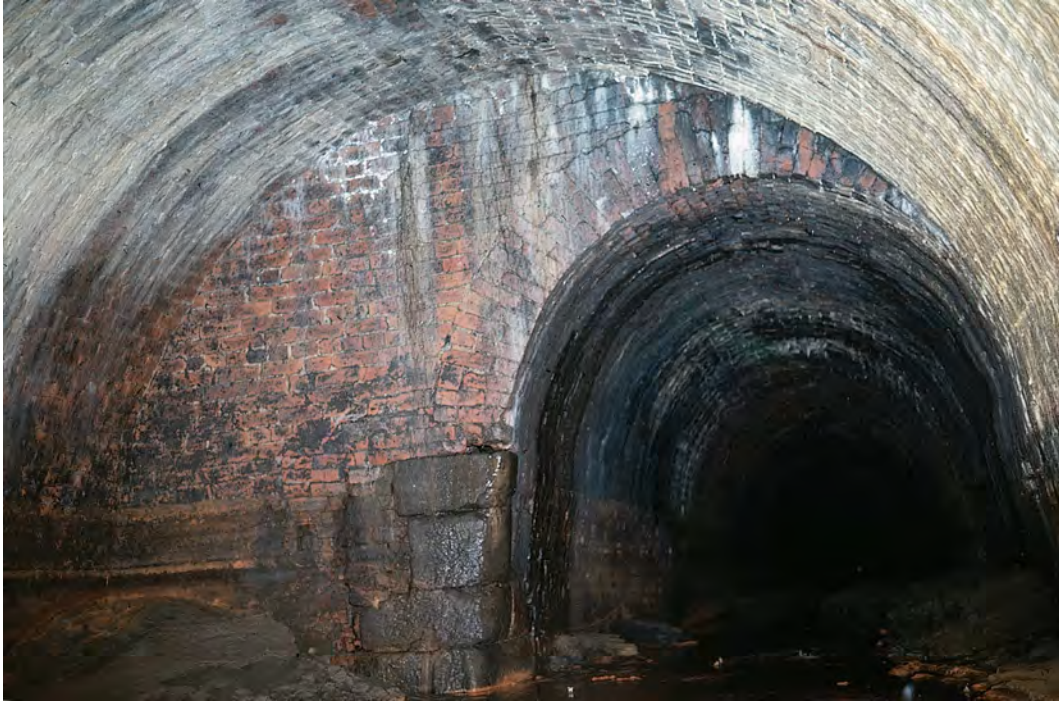
Figure 10: East facing internal elevation of the wide hole, showing stone quoins protecting the projecting west corner, looking west (after Witter 1979, image 11), © Robin Witter, reproduced with permissions
