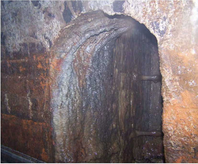
Figure 15: Entrance to narrowed vertical shaft, showing iron rungs (after Cordon 2006, image 82), © Tina Cordon, reproduced with permissions
