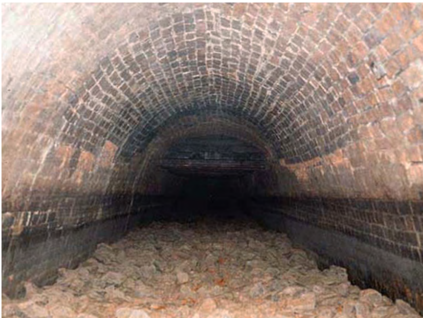
Figure 7: Limestone infill in the Butterley Tunnel, (after Witter 1979, image 13) © Robin Witter, reproduced with permissions
