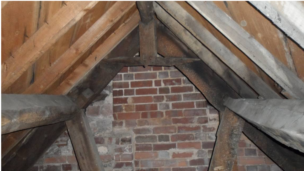
Figures 4c/d: Views of wall framing in 15 Stepcote Hill (top) and roof to 16 Stepcote Hill (bottom; photographs Robert Howard)
