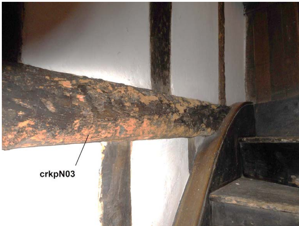
Figure 10: View of the elm mid-rail at the west end of the east section of the north-west range, sampled as crkpN03 (photograph Martin Bridge)
