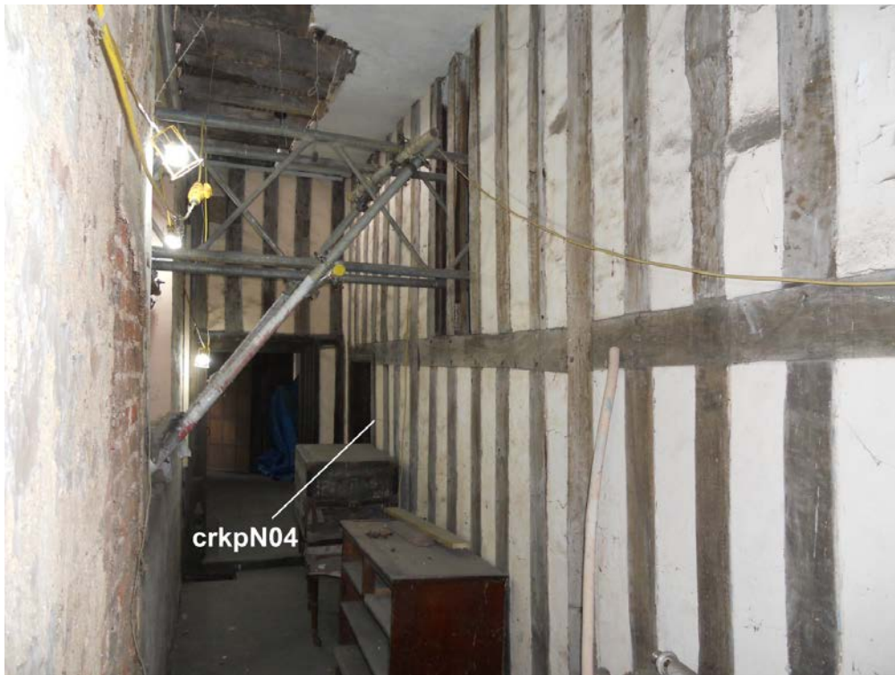
Figure 9: View looking west along the ground floor corridor to the north-west range, showing the position of the timber sampled as crkp04 (photograph Martin Bridge)
