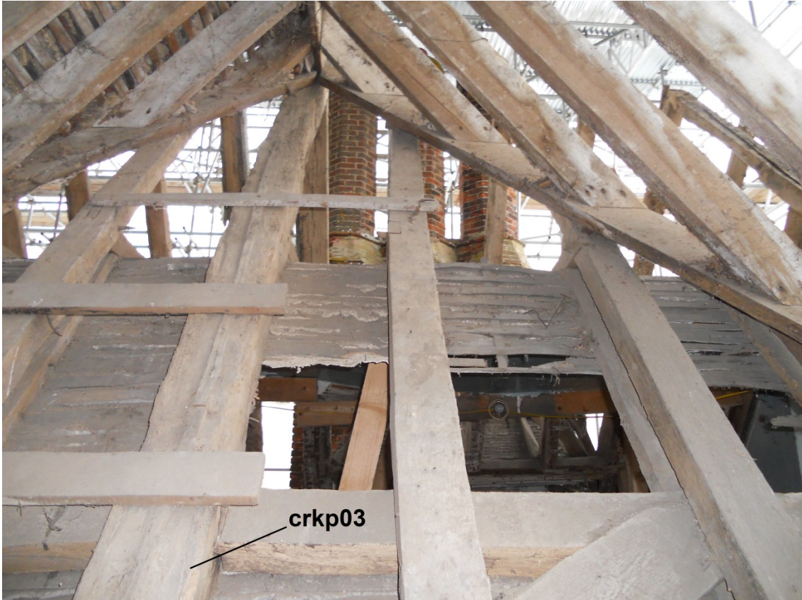
Figure 5: View of the east end bay of the north range, looking north, showing the south principal rafter sampled for dendrochronology (photograph Martin Bridge)
