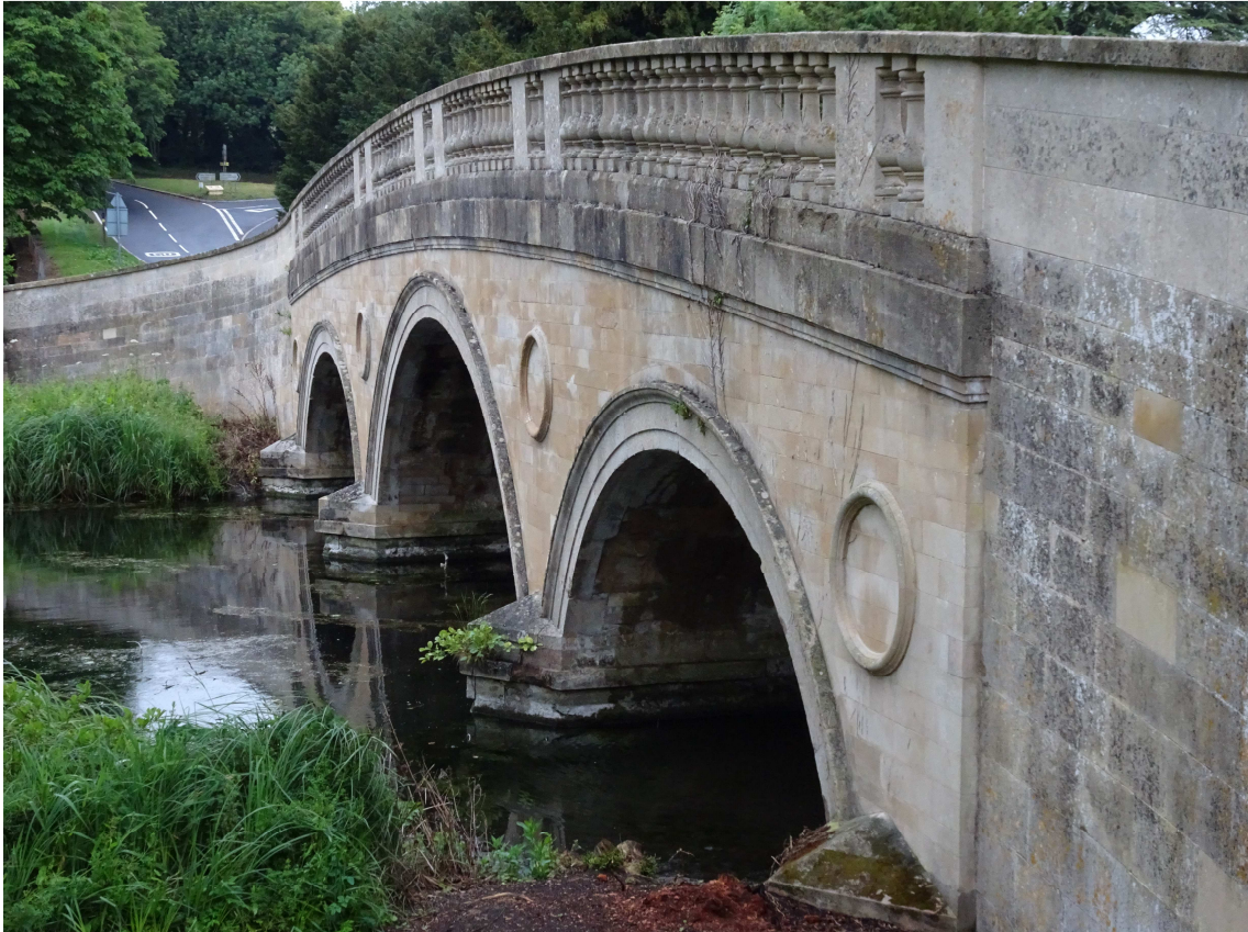
Plate 2 view of the Adam Bridge from the east bank of the Cam looking west.
