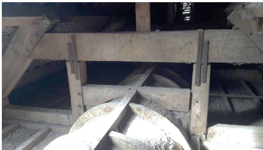
Figure 4: Roof and truss 3. Photograph taken from the east and at above ceiling level (Robert Howard)
