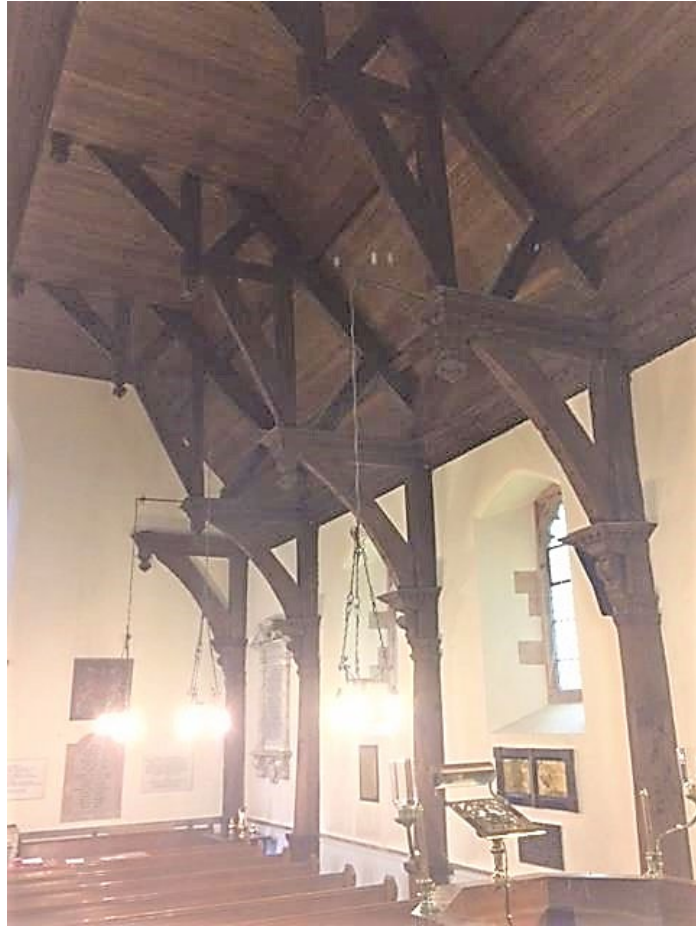
Figure 3: The roof, with truss 3 in the foreground. Photograph taken from the south-east (Robert Howard)
