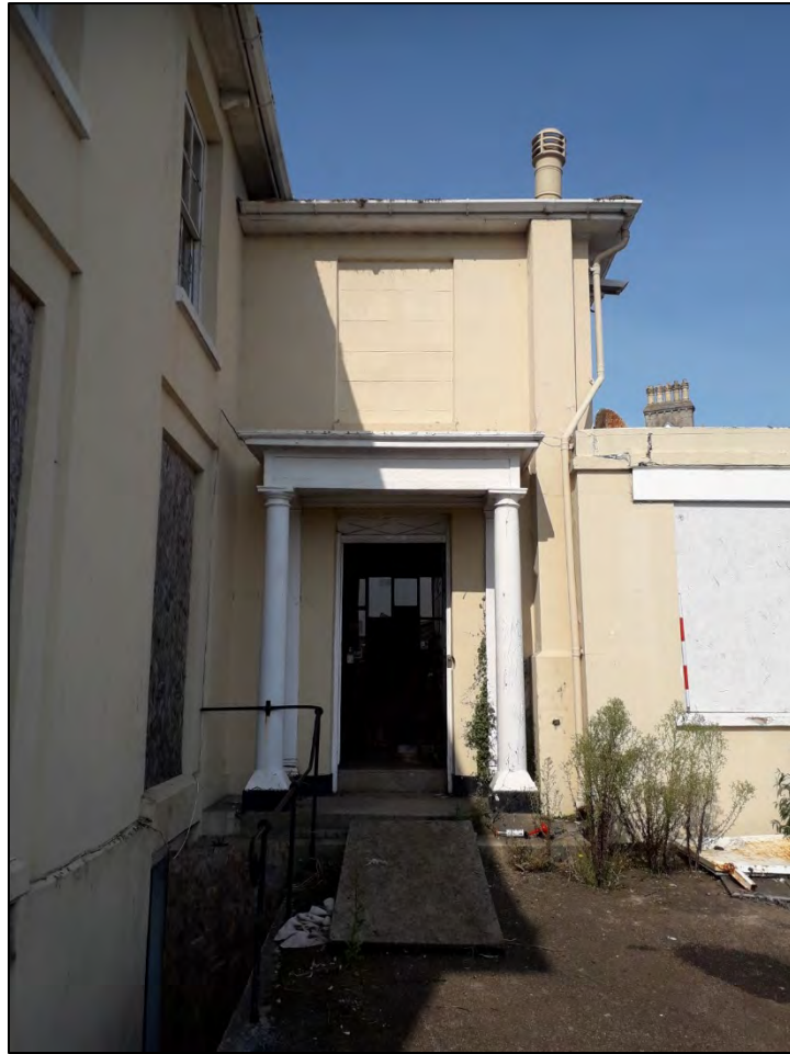
Plate 7: 1 Penrose Terrace, south elevation of north (side) wing, view to the North, 1m scale.
