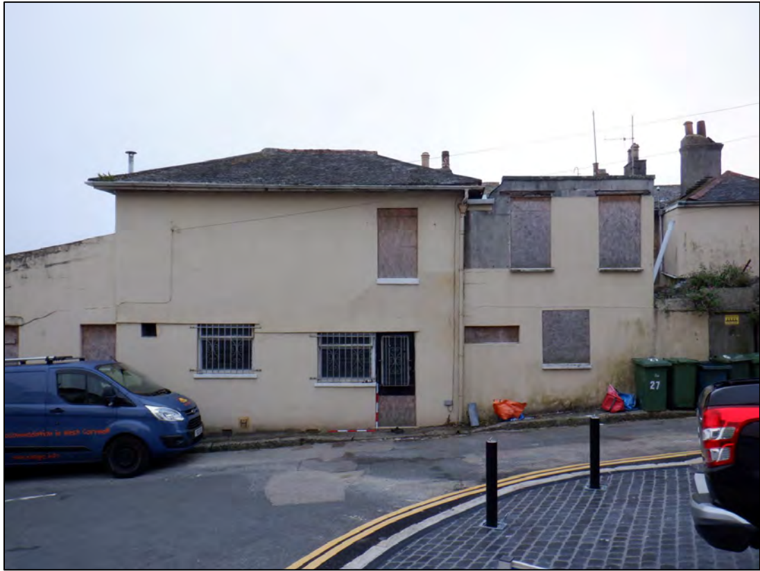
Plate 13: 1 Penrose Terrace, north elevation of north wing, view to the south, 2 x 1m scale.
