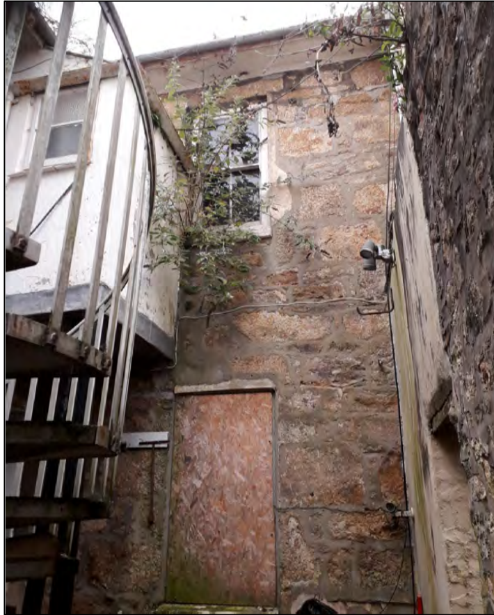
Plate 15: 1 Penrose Terrace, north elevation of south wing, view to the south, 1m scale.
