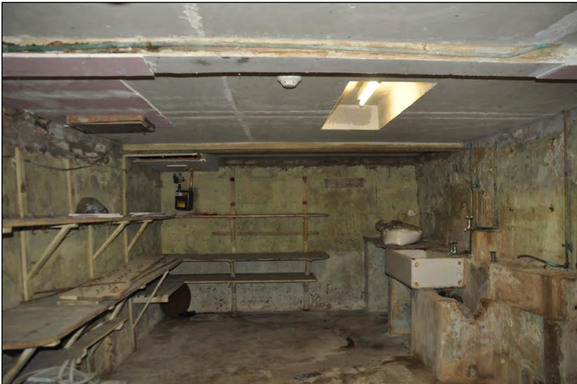
Plate 95: 1 Penrose Terrace, Room 1B7, view to the E. Image supplied by CAD Heritage.
