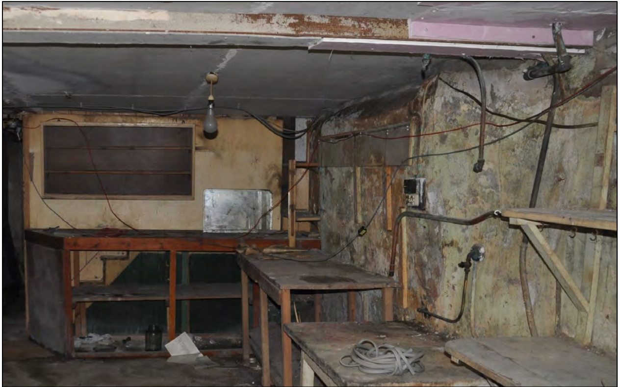
Plate 100: 1 Penrose Terrace, Room 1B7, view to the WNW. Image supplied by CAD Heritage.
