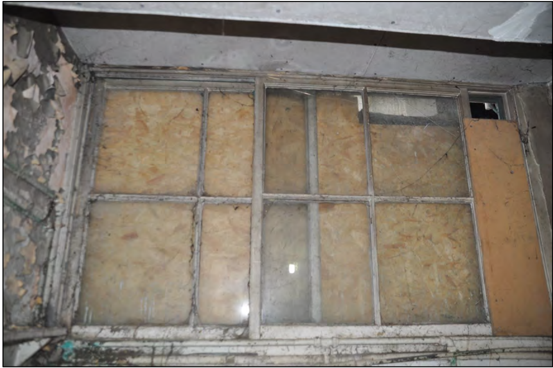
Plate 82: 1 Penrose Terrace, Room 1B3, view to the N. Image supplied by CAD Heritage.
