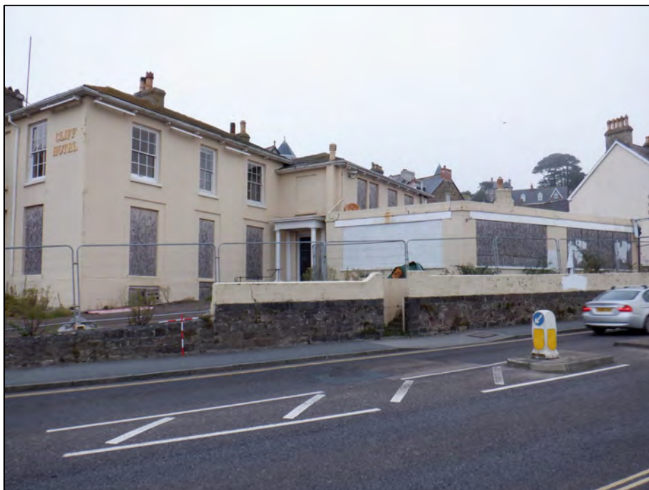
Plate 8: 1 Penrose Terrace, south elevation of NE Annexe, view to the NNW, 2 x 1m scale.
