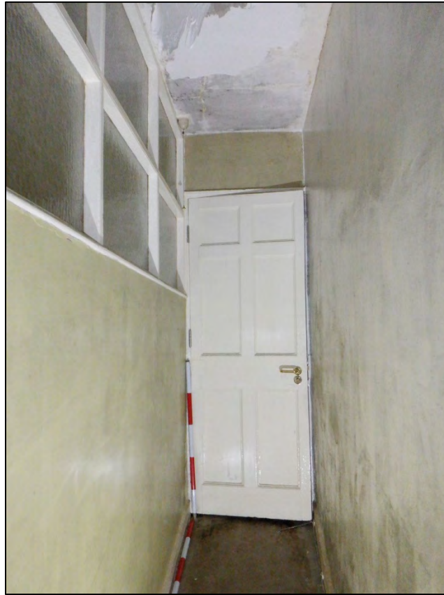
Plate 142: 2 Penrose Terrace, Corridor east of Room 2G7, view to the N. 2 x 1m scale.
