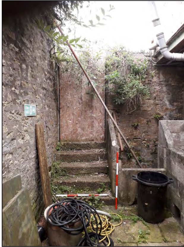
Plate 108: 1 Penrose Terrace, External Rear Yard, view to the N. 2 x 1m scale.
