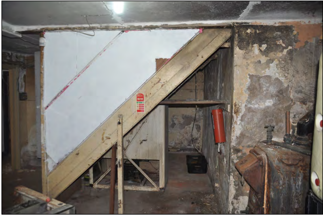
Plate 80: 1 Penrose Terrace, Room 1B3, view to the S. Image supplied by CAD Heritage.
