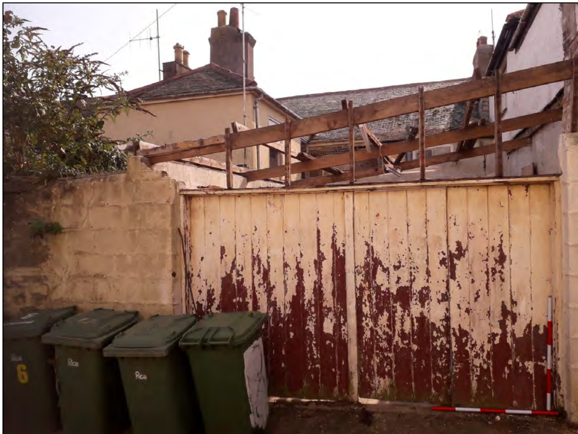
Plate 119: 2 Penrose Terrace, North Facing Elevation, view to the SSE. 2 x 1m scale.
