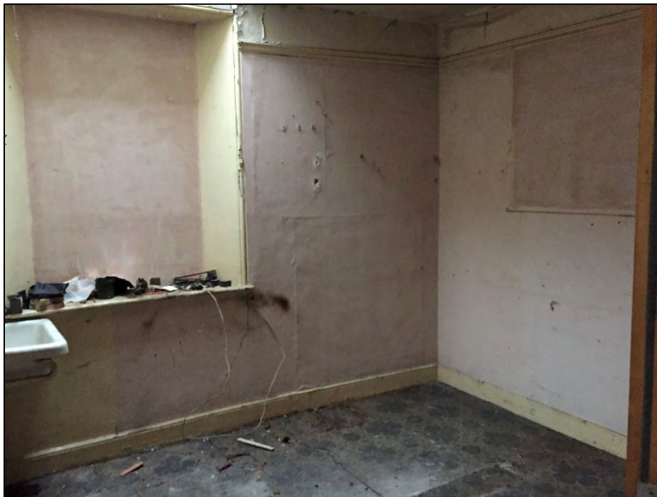
Plate 67: 1 Penrose Terrace, Room 1F12, view to the NE. Image supplied by CAD Heritage.
