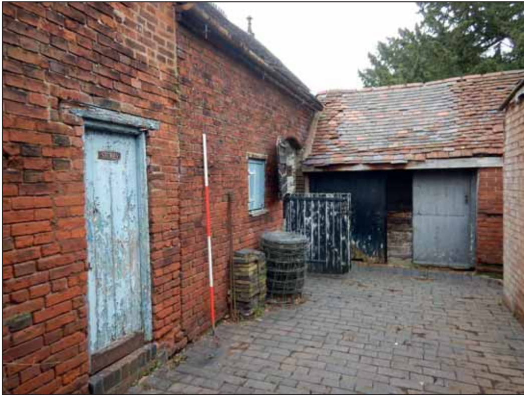
Plate 23: South Facing Elevation of the east end of the main barn and Dog Kennels, Looking ENE. 2m scale.
