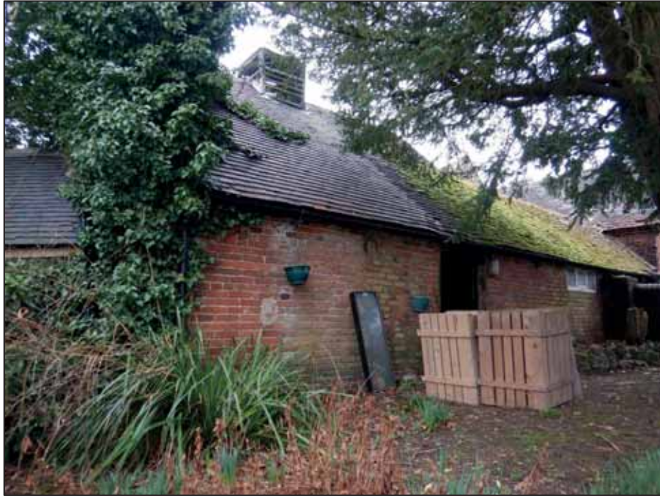
Plate 19: East Facing Elevation of the S end of the East Wing, looking NW.
