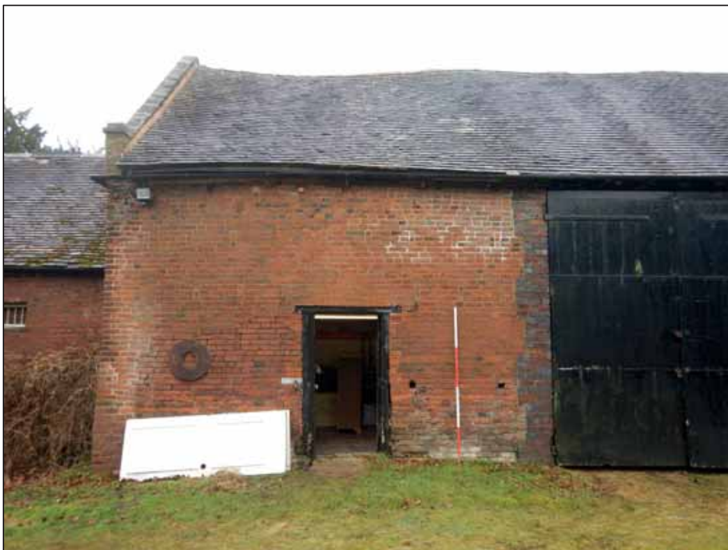
Plate 4: North Facing Elevation of the east end of the Main Barn, looking S. 2m scale.
