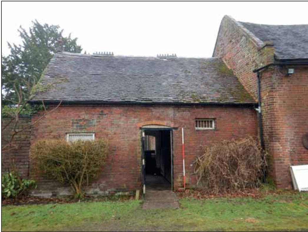
Plate 3: The North Facing Elevation of the Dog Kennels, looking S. 2m scale.
