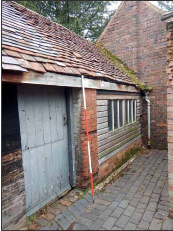
Plate 29: West facing elevation of the East Wing (central section), looking SSE, 2m scale.
