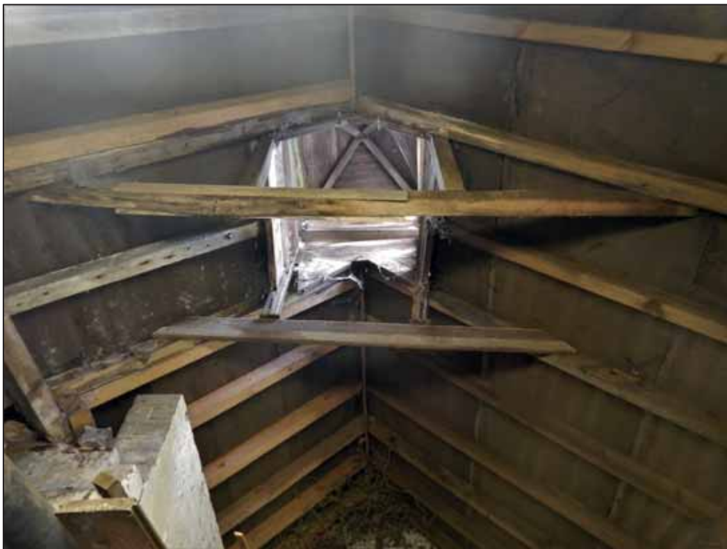
Plate 58: East Wing, Shed, roof structure including internal view of beehive vent. view to the S.
