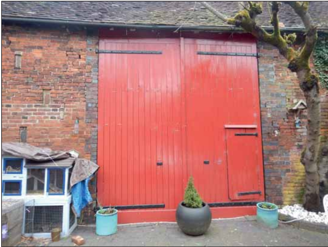
Plate 25: South Facing Elevation of the Main Barn, central double doors, looking N.
