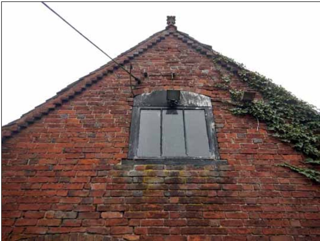
Plate 16: East Facing Elevation of the east gable of the Dog Kennels, looking W.
