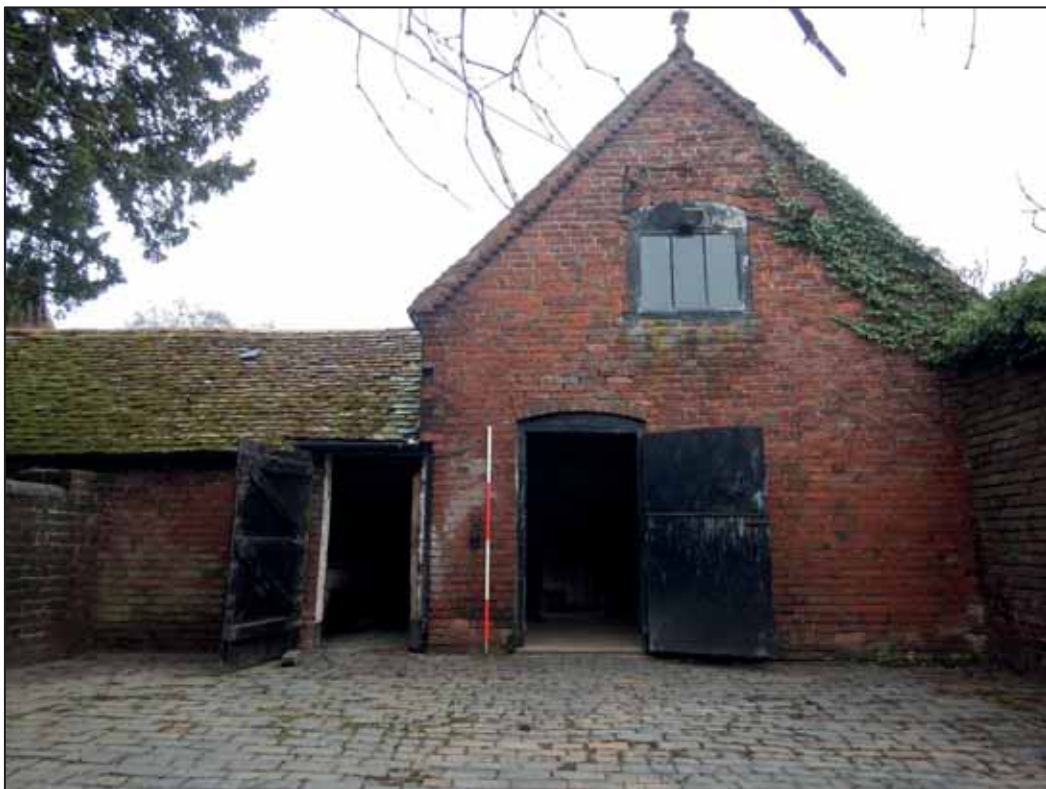
Plate 10: East Facing Elevation of the Dog Kennels and the N end of the East Wing, looking W. 2m scale.
