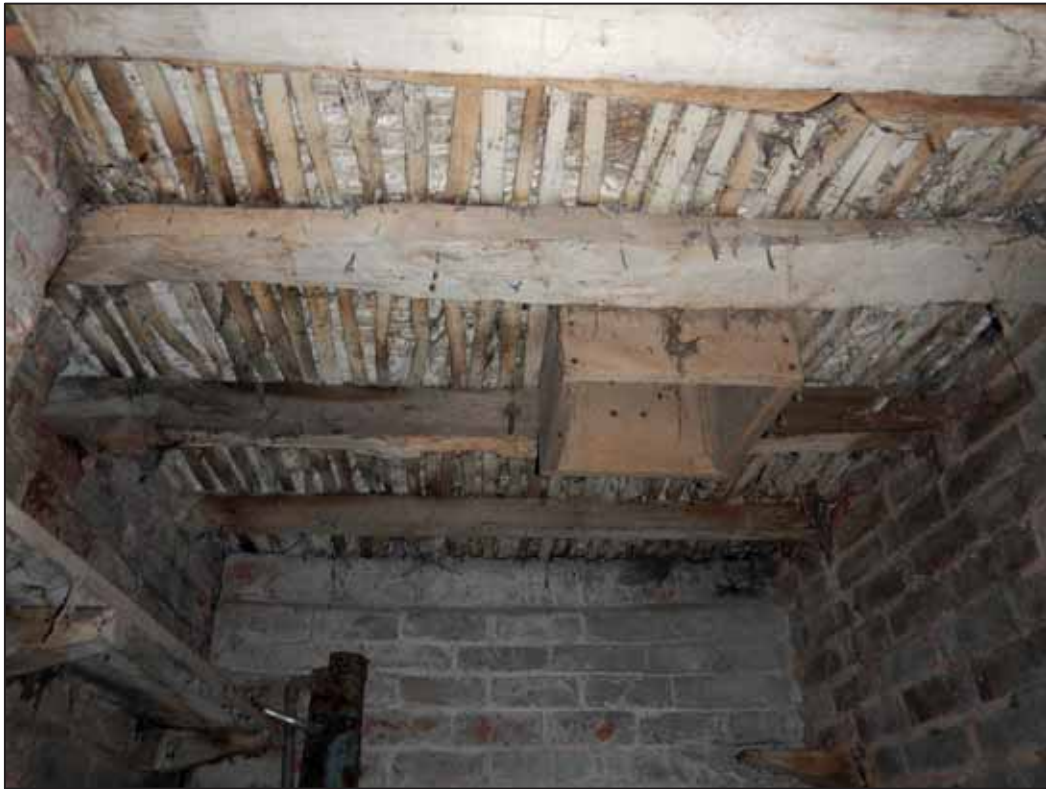
Plate 41: Main Barn, small store, showing original joists, lathes and former grain chute. looking E.
