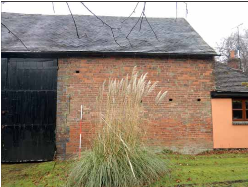
Plate 6: North Facing Elevation of the west end of the Main Barn, looking S. 2m scale.
