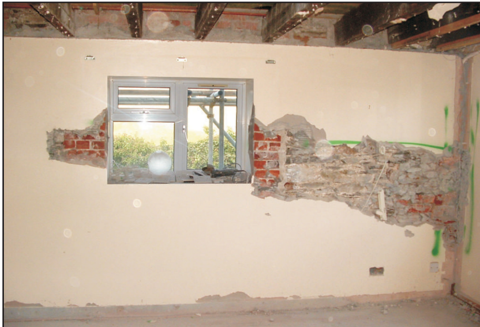
Fig. 26 North range: ground floor, E room showing blocking of splays of early window, with scar of demolished E gable wall to right.
