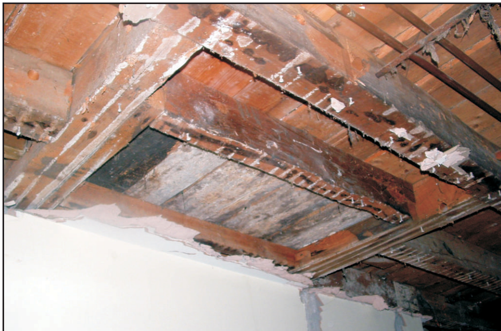
Fig. 14 Assembly of first-floor joists showing trimmers, joist box, and thick boards to support first-floor fireplace.
