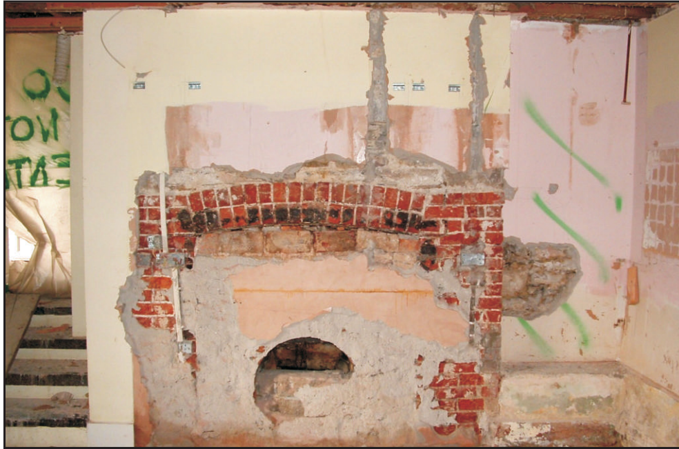
Fig. 13 The hall fireplace. Note iron bar supporting the lintel, wooden blocks for original fireplace surround, area of sooted brickwork exposed within the former surround, and blocking for 19th-century hob grate.
