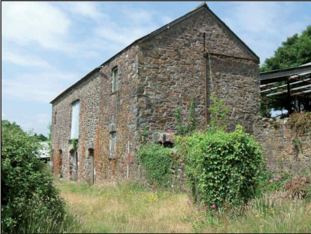
Photo. 1 South and east elevations of the barn showing yard wall in foreground, looking northwest. 2m scale.
