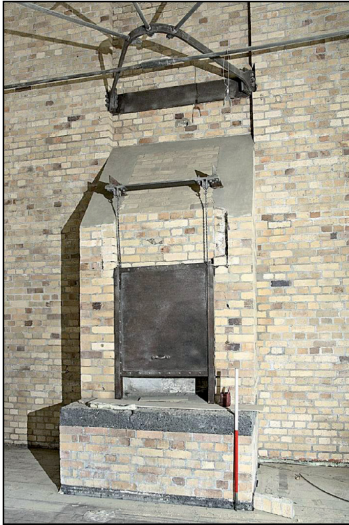
Photo. 9 Room F7, showing hearth in the north partition wall, looking north. 1m scale.
