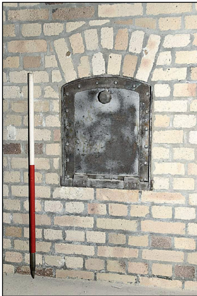
Photo. 3 Room G1 (entrance hall) showing delivery hatch in west wall, looking west. 1m scale.
