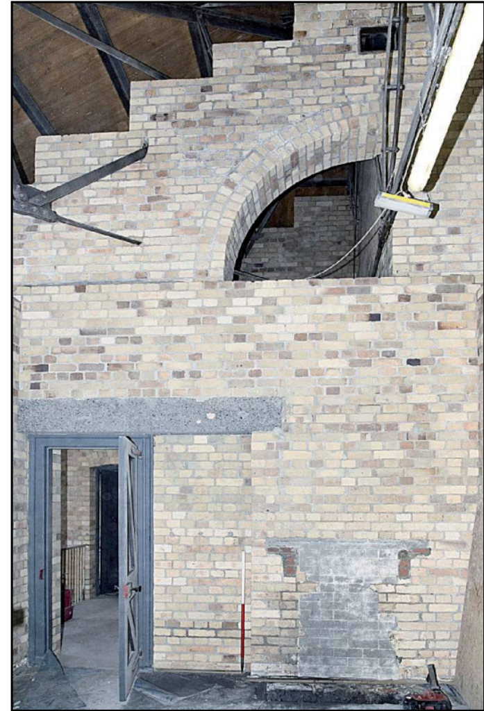
Photo. 8 Room F2, showing blocked fireplace, door and stepped and arched masonry containing flues, looking east. 1m scale.
