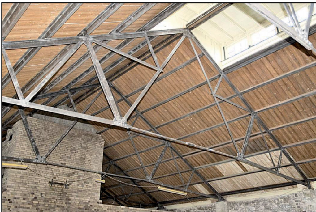
Photo. 10 View of the roof trusses and skylight above room F6, looking north-east.
