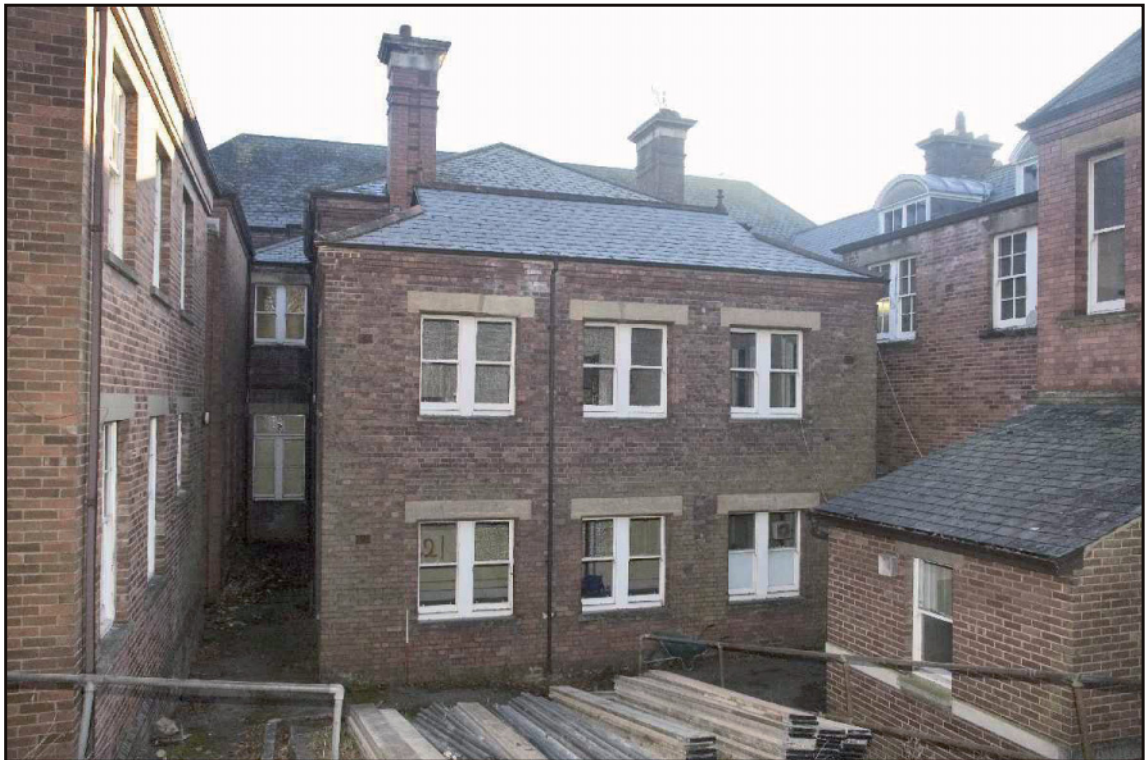
Photo. 2 The north west wing, showing the west elevation, looking east. 1m scale.
