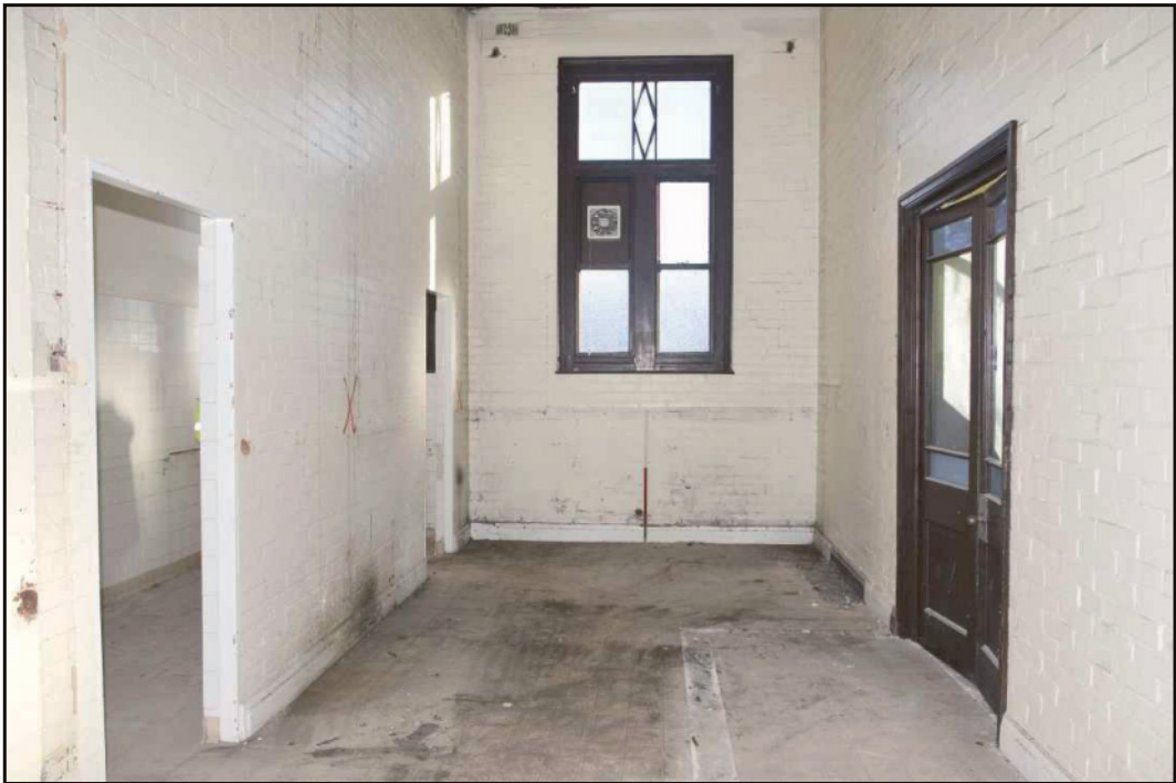
Photo. 11 The changing room and showers in the 1935 extension, looking east. 1m scale.
