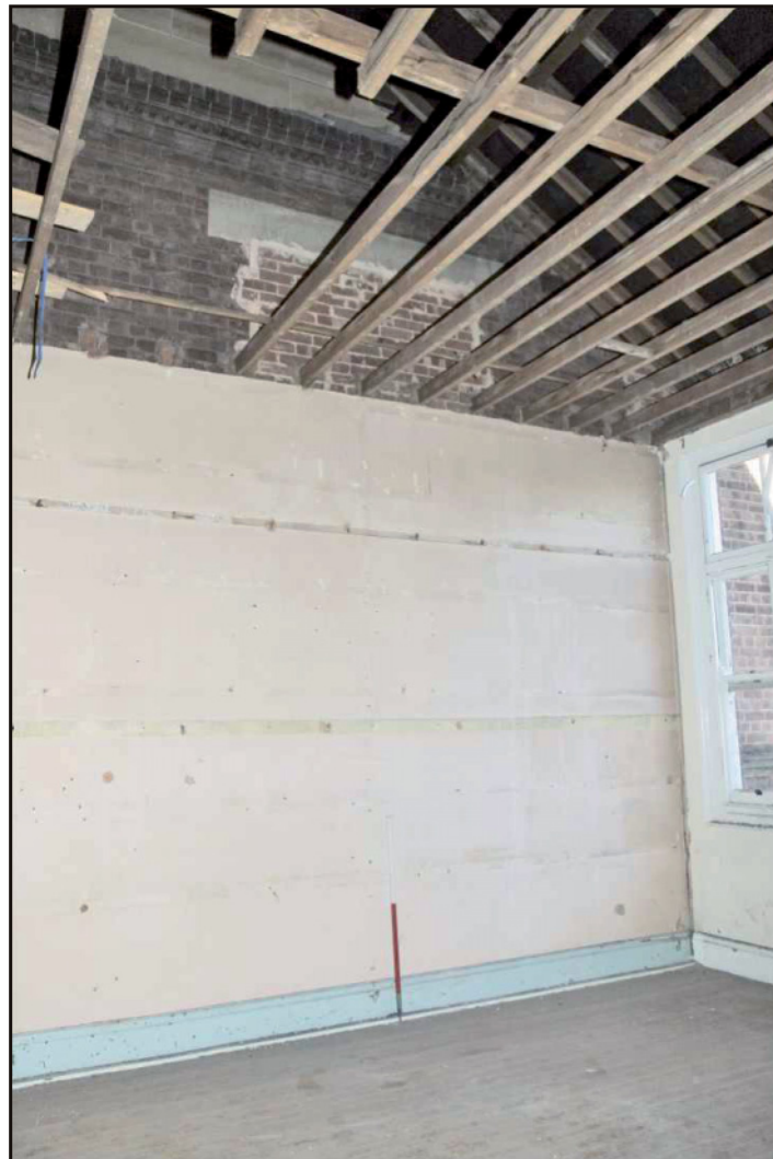
Photo. 11 The first floor of the 1935 extension, showing blocked window in the original school building, looking north east. 1m scale.
