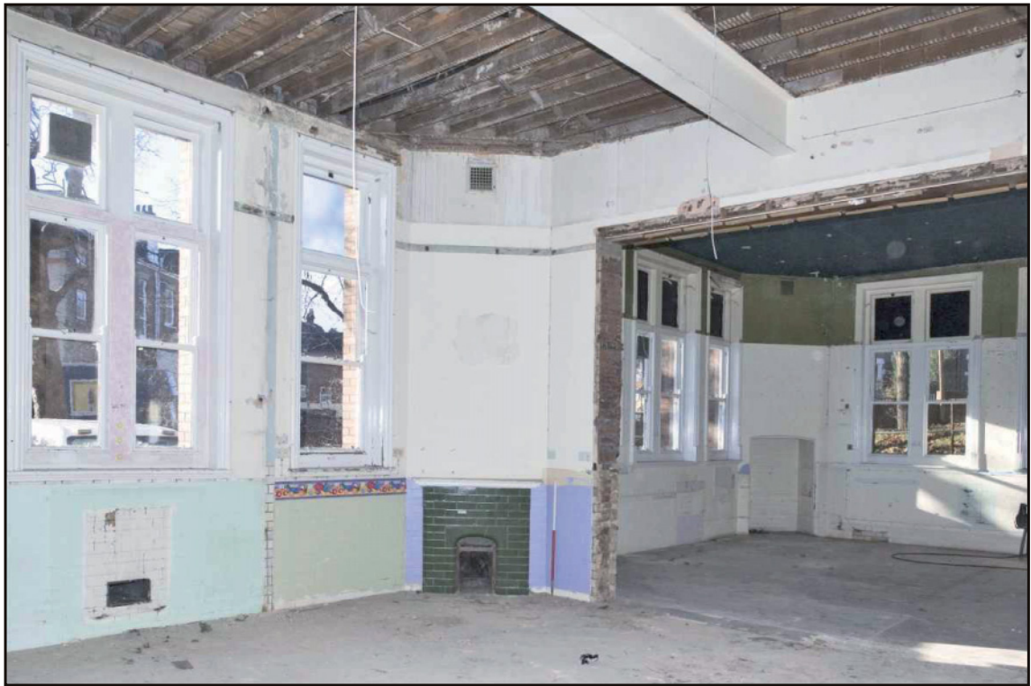
Photo. 9 The 1908 ground floor science rooms, showing fireplaces and tiled walls, looking west. 1m scale.
