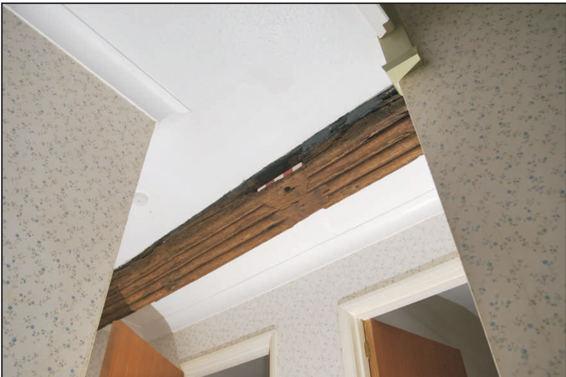
Photo 6 The reused beam from an intersecting beam in the cottage, looking southeast. 0.25m scale.
