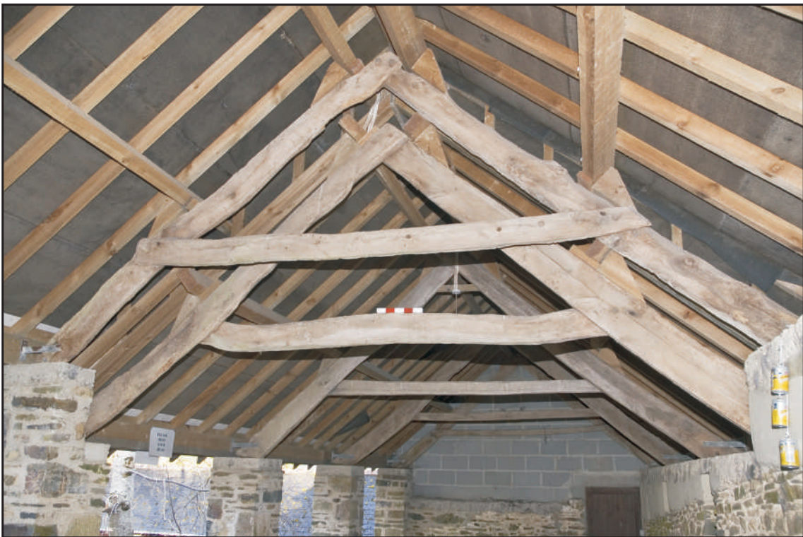
Photo 8 The roof trusses in the southern range shippon, looking northeast. 0.25m scale.
