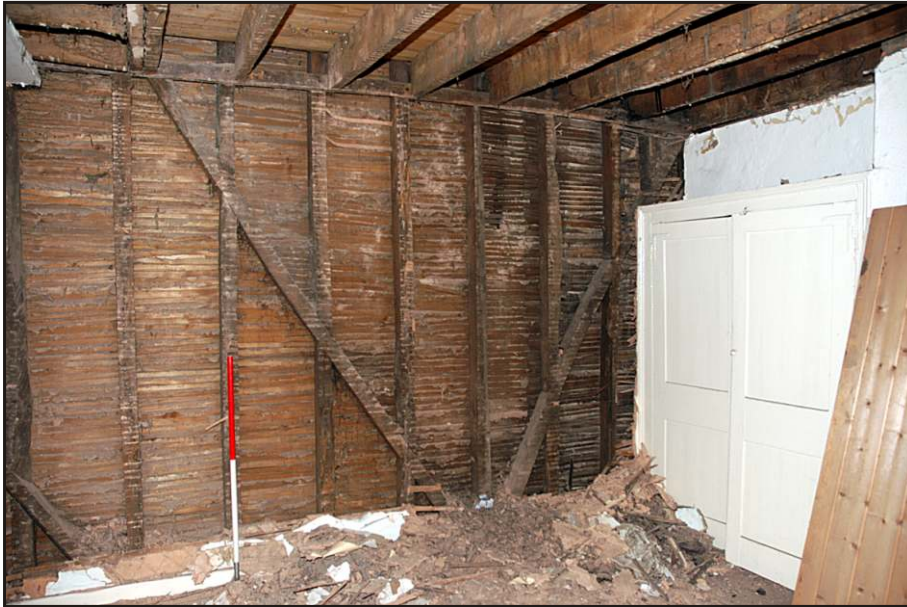
Fig. 19 View of the south-eastern room at third-floor level showing the construction of the late 18th-century upper storeys of the building. The ceiling joists are supported by a trimmer nailed against the studwork of the adjoining building, which is unrelated to them structurally. The late 18th-century fitted cupboard is also shown.
