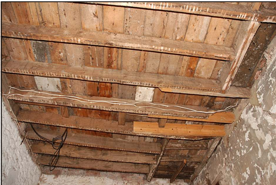
Fig. 12 Detail of the ceiling in the extension showing the provision for a staircase.
