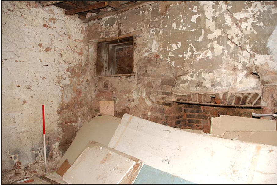
Fig. 11 View of the room within the extension showing the fireplace and window in the plastered south-east wall and the city wall forming the north-east wall.
