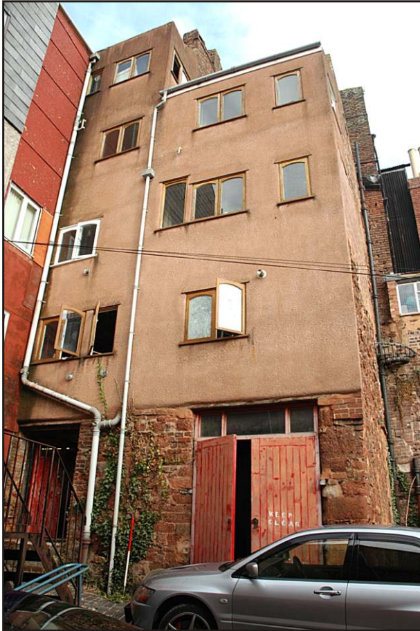
Fig. 5 View of the house from Rackclose Lane showing the exposed parts of its south-western façade.
