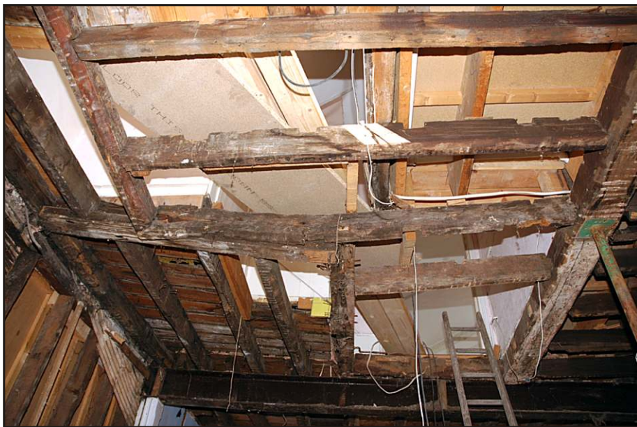
Fig. 15 Detail of the ceiling structure seen from the second floor, showing the crude infilling of the void of the 18th-century staircase and the poor structural condition of the building.
