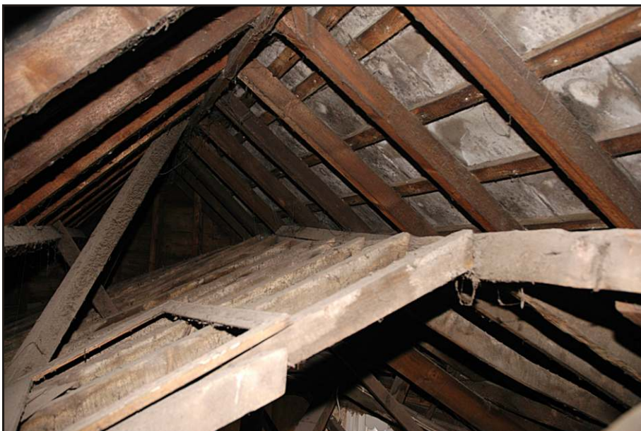
Fig 20 Detail of the roof space showing the superimposed roofs of the north-western parts of the building.
