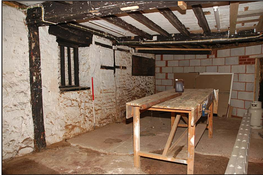
Fig. 7 interior of the ground-floor room in the main building, looking north west showing the blocked window and doorway in the south-western wall and the modern partition hiding the relationship of the house and the viaduct.
