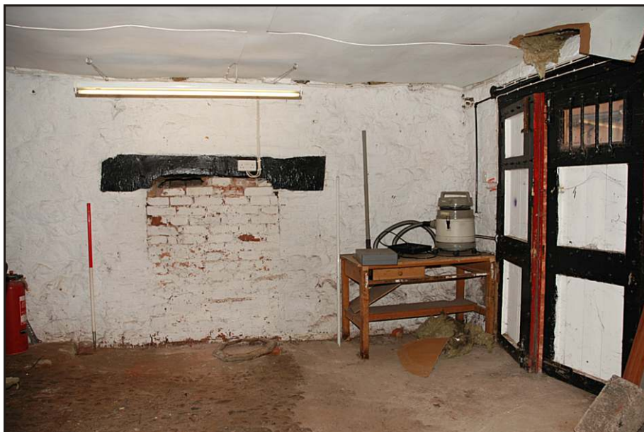
Fig. 8 View of the south-eastern end of the room showing the blocked 17th-century fireplace.
