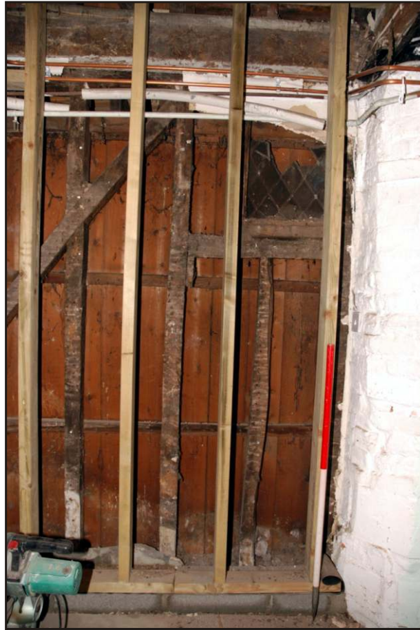
Fig. 14 Detail of the small window discovered at first-floor level in the south-west wall, showing the character of the timber framing at this level.
