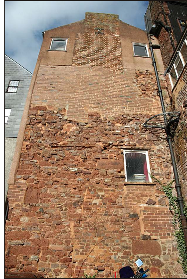
Fig. 6 View of the gable end of the extension showing the brick chimney inserted at ground-floor level (bottom centre), the refacing of the second-floor elevation (centre, top) and the later 18th-century fabric enveloping the chimney stack above.
