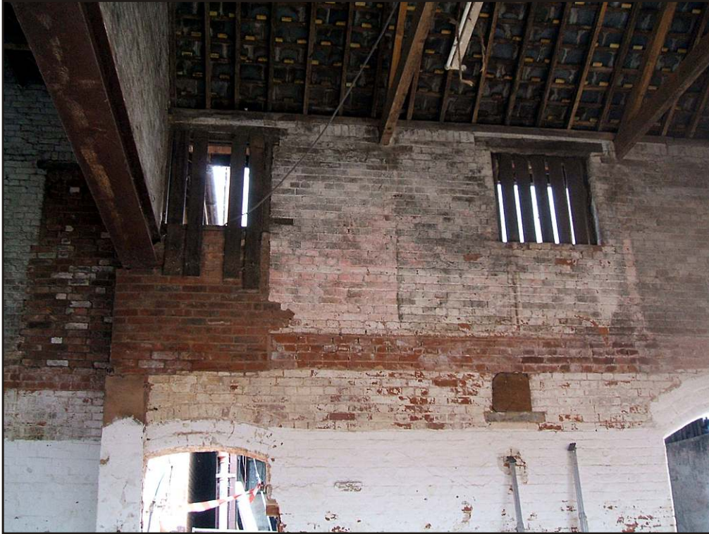
Plate 11 Barns 7 and 8, south (inside) elevation showing removed wall (left) and beam (right) looking southeast.
