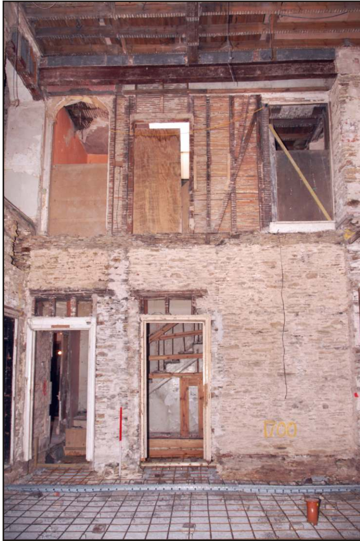
Fig. 23 View of the mid 19th-century partition between the service stair and the rooms in the service wing, showing later 19th-century alterations to the openings and the character of the structure.
