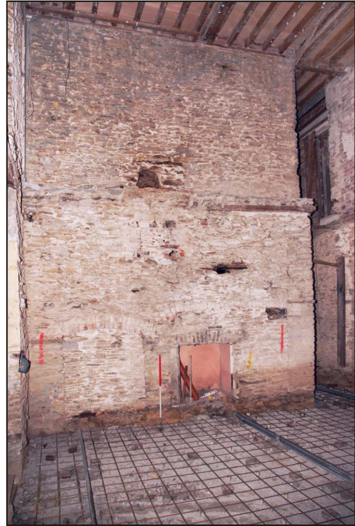
Fig. 24 View of the fireplaces in the eastern wall of the old kitchen, showing the blocked openings and traces of the earlier roofline of the range as a wall scar above.
