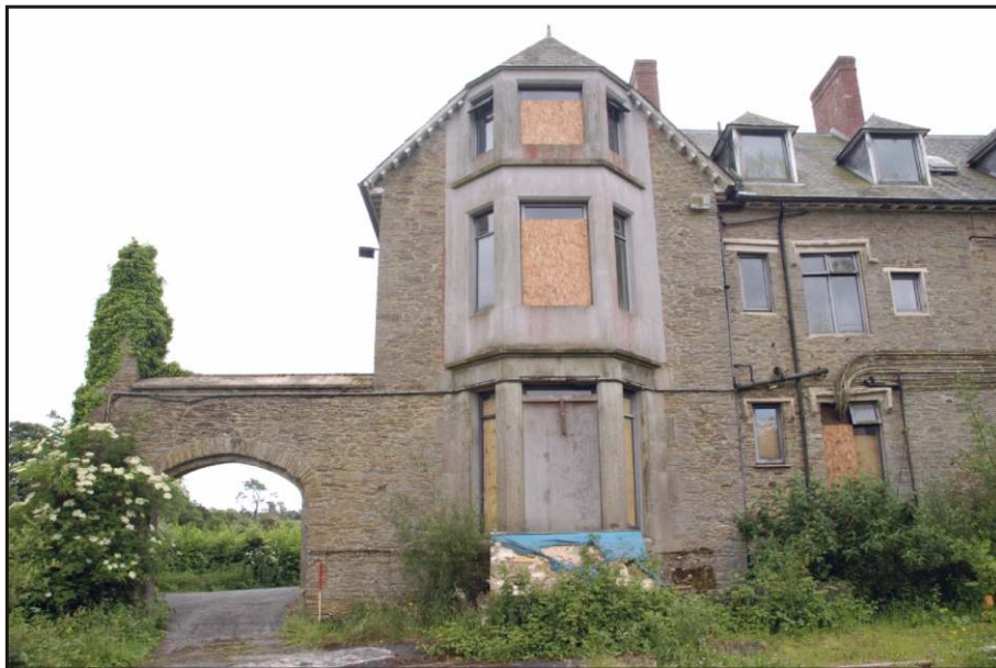
Fig. 15 View of the north elevation of the main house showing the rear view of the archway and the inserted bay window. A vertical break in the masonry of the upper floor may be discerned on the extreme right.
