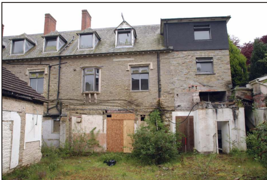
Fig. 16 The western end of the north façade of the service range, showing the extent of 20th-century alterations.
