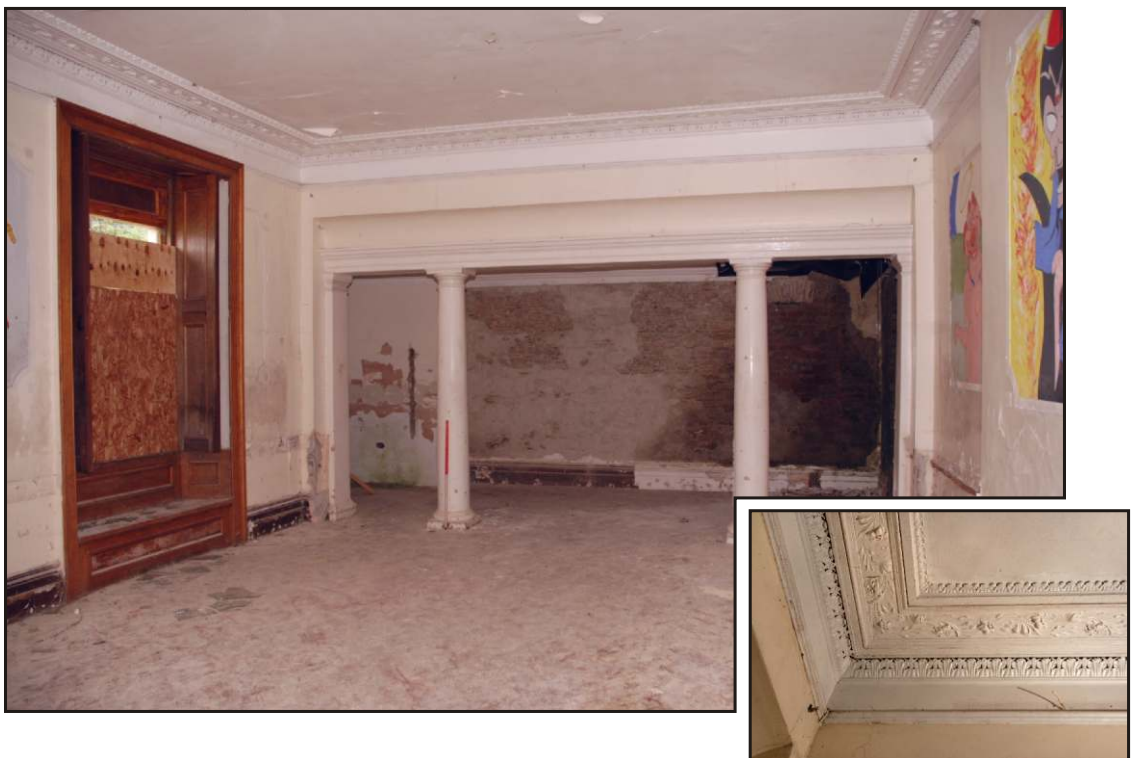
Fig. 22 The large ground-floor room in the centre of the southern part of the house, showing the window shutters, screen of columns and plaster decorations (detail of cornice inset).
