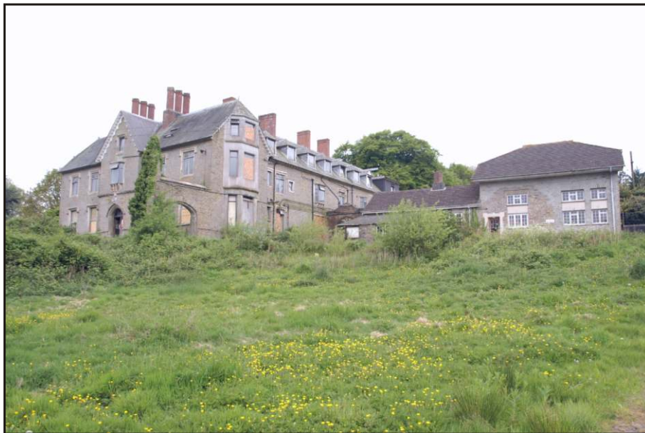
Fig. 6 View of the house from the north-east, showing the condition of the building prior to refurbishment and the heavily altered service ranges to the north.
