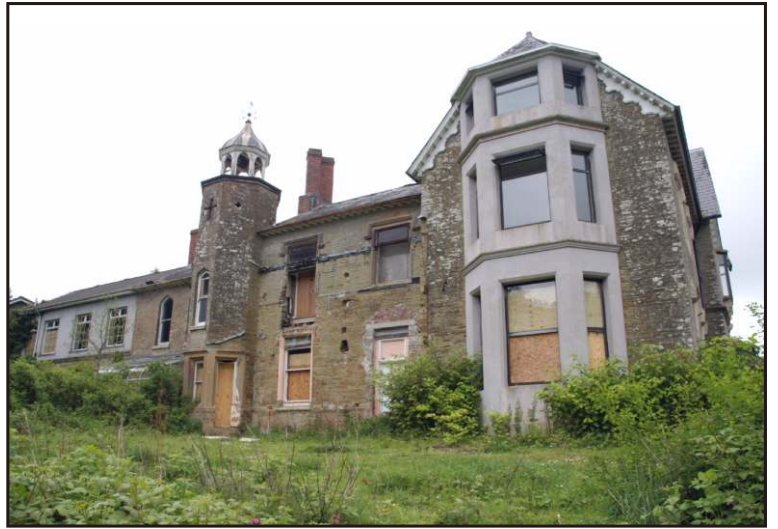
Fig.12 View of the south façade of the house showing alterations made since c.1869 (compare Fig.5).
