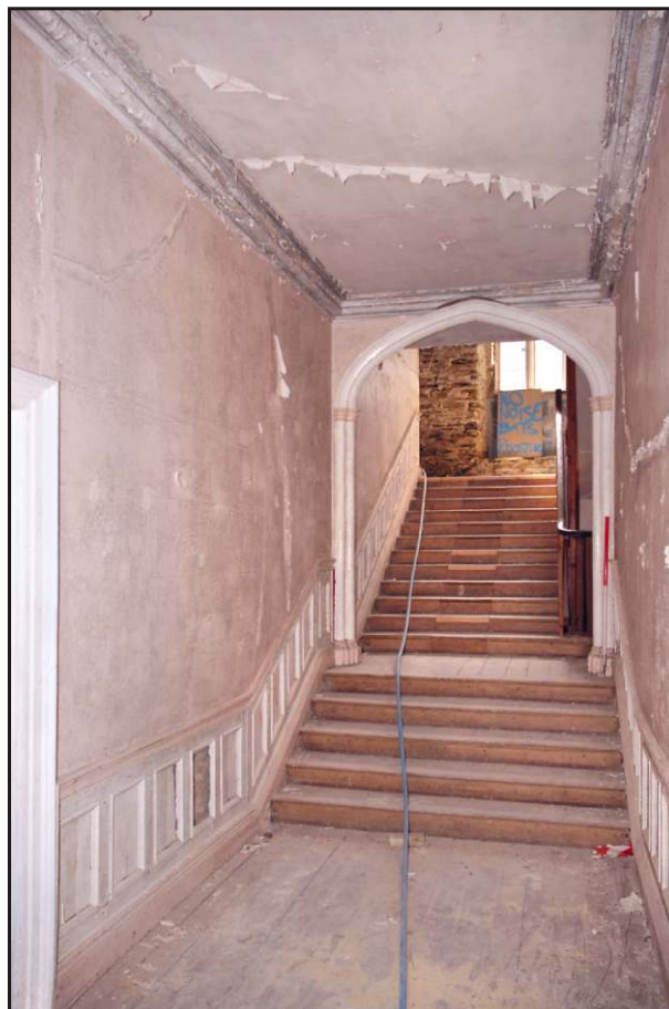
Fig. 20 The main corridor, looking west towards the foot of the staircase. The collision between the top of the archway and the cornice and the widened staircase can clearly be seen.
