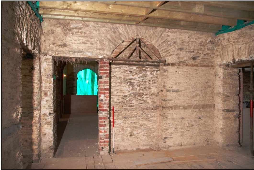
Fig. 28 View looking east in the central first-floor room, towards the main stairs and landing, showing the arched alcove as revealed by the building works, and 19th-century attempts to disguise it.
