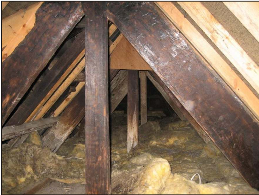
Fig. 32 Evidence of charring and fire damage to the ?19th-century roofs of the northern part of the house following a minor 20th-century fire.
