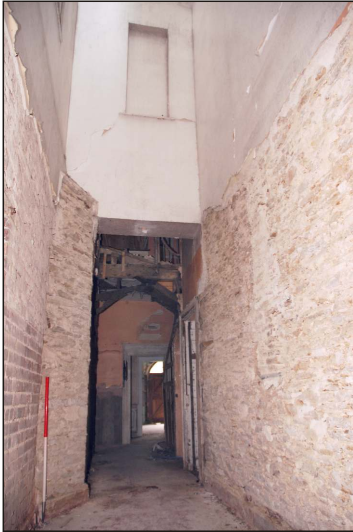
Fig. 25 The corridor or light well alongside the old kitchen, looking towards the service stair, showing blocked windows on the first floor and an enigmatic chase in the wall (right).
