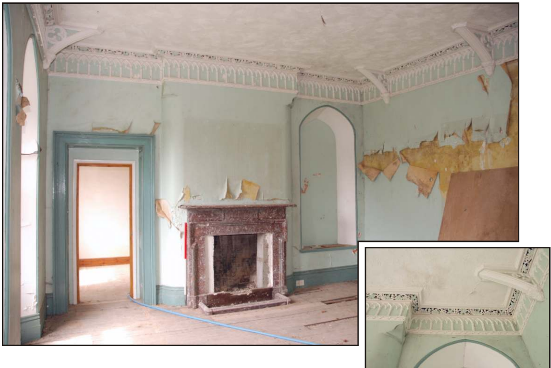
Fig. 29 View of the first-floor ballroom looking east, showing the marble fireplace, plasterwork and blocked windows and openings into the conservatory beyond (detail of the plasterwork inset).
