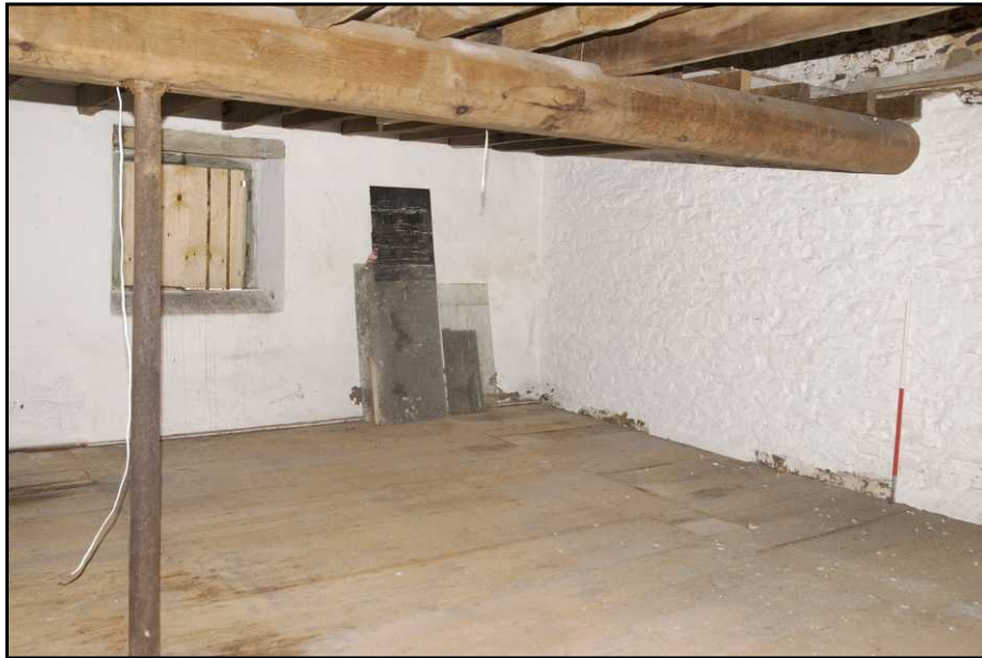
Plate 5 View of the first floor showing a ship's mast reused as a beam, looking south-west. 1m scale.
