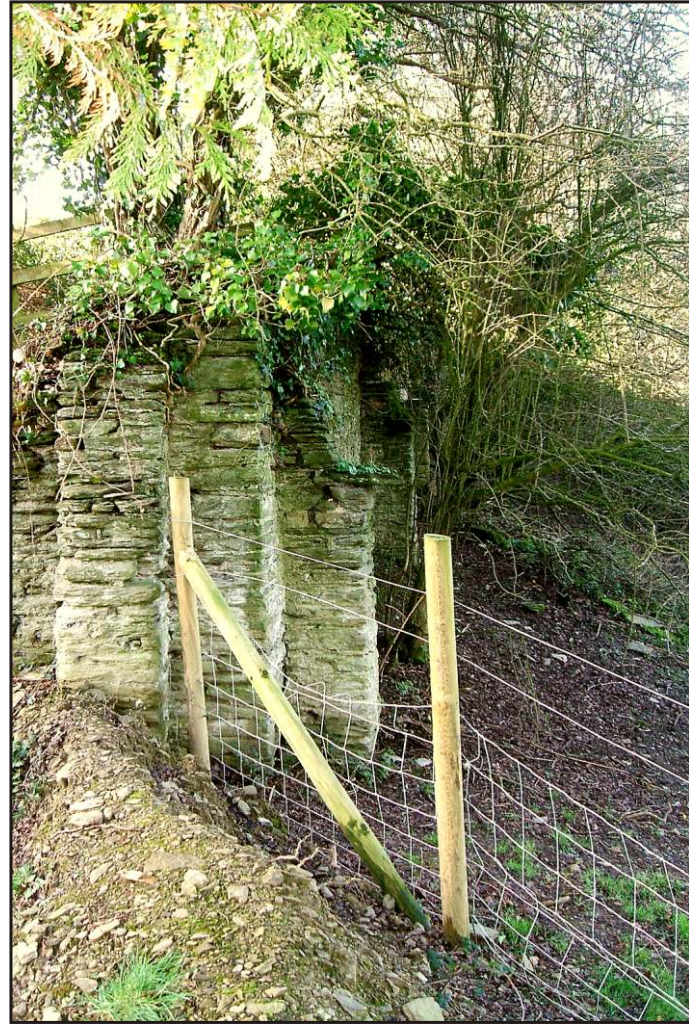
Pl. 6 General view of stone retaining wall at the front of building terrace. Looking north-west.
