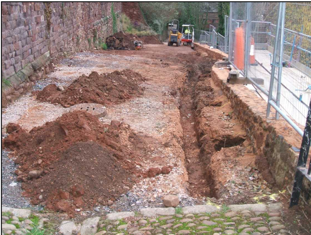
Plate 2 Cricklepit Street, showing extent of ground reduction and location of service trench, looking south-east.
