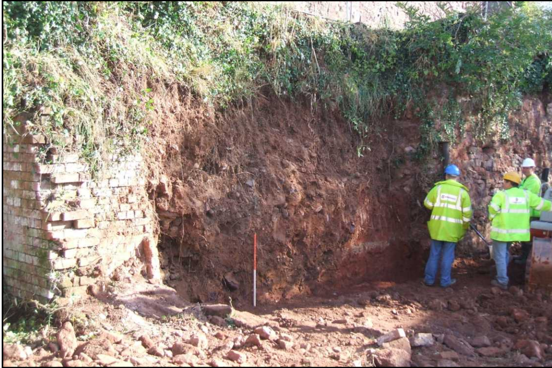
Plate 1 Excavation for new retaining wall showing infill deposits overlaying natural, looking north-east. 1m scale.
