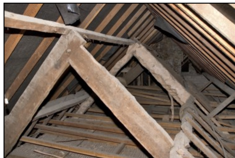
Fig. 19 View within the roof showing the apex of the early roof beneath the modern roof structure.
