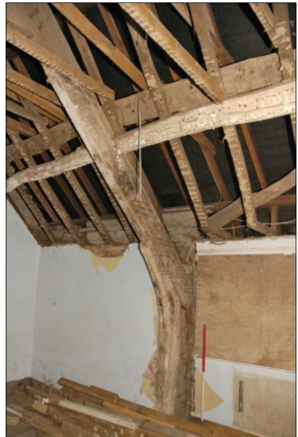
Fig. 15 Detail of a jointed cruck in the northern room on the first floor.
