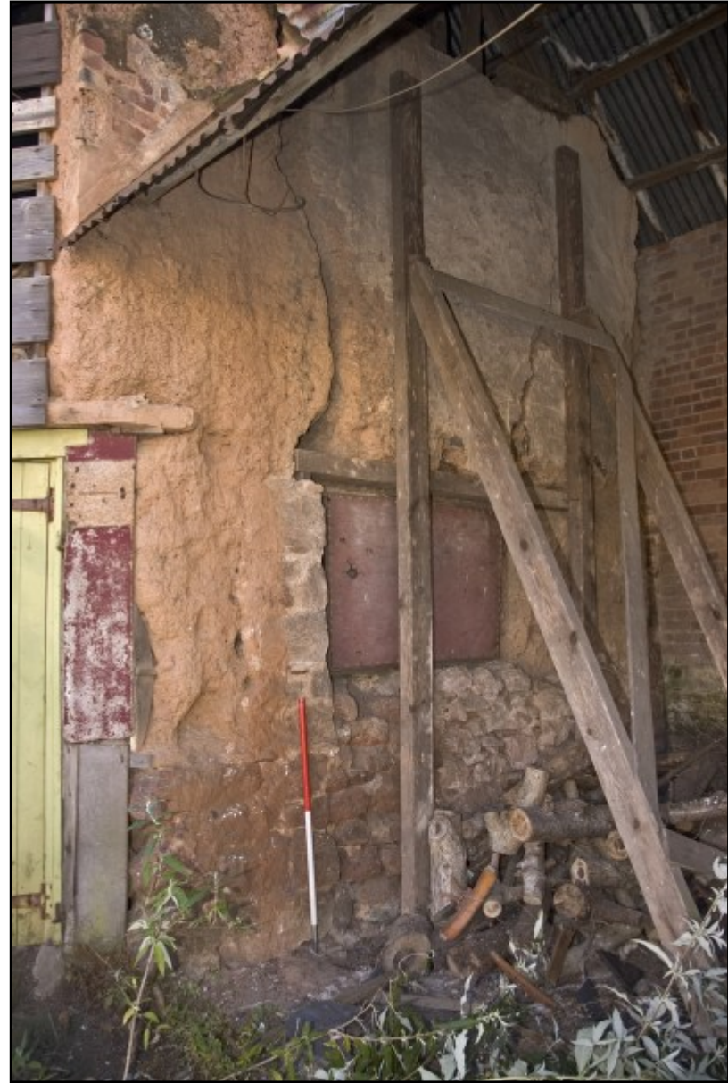
Fig. 22 Detail of the west gable wall of the stable prior to rebuilding, showing its parlous condition.
