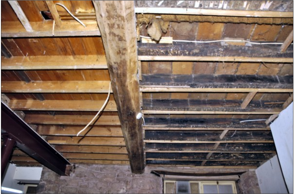
Fig. 13 View of the ceiling of the hall after removal of the plaster showing the extent of modern interventions (left).
