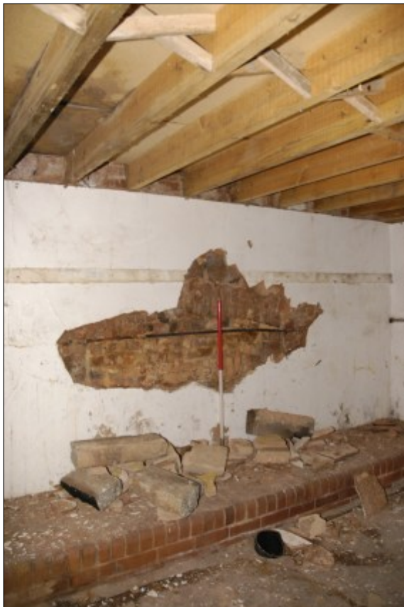
Fig. 14 View of the west wall in the north-western cross wing during stripping, showing the blocked kitchen fireplace and the modern first-floor structures.
