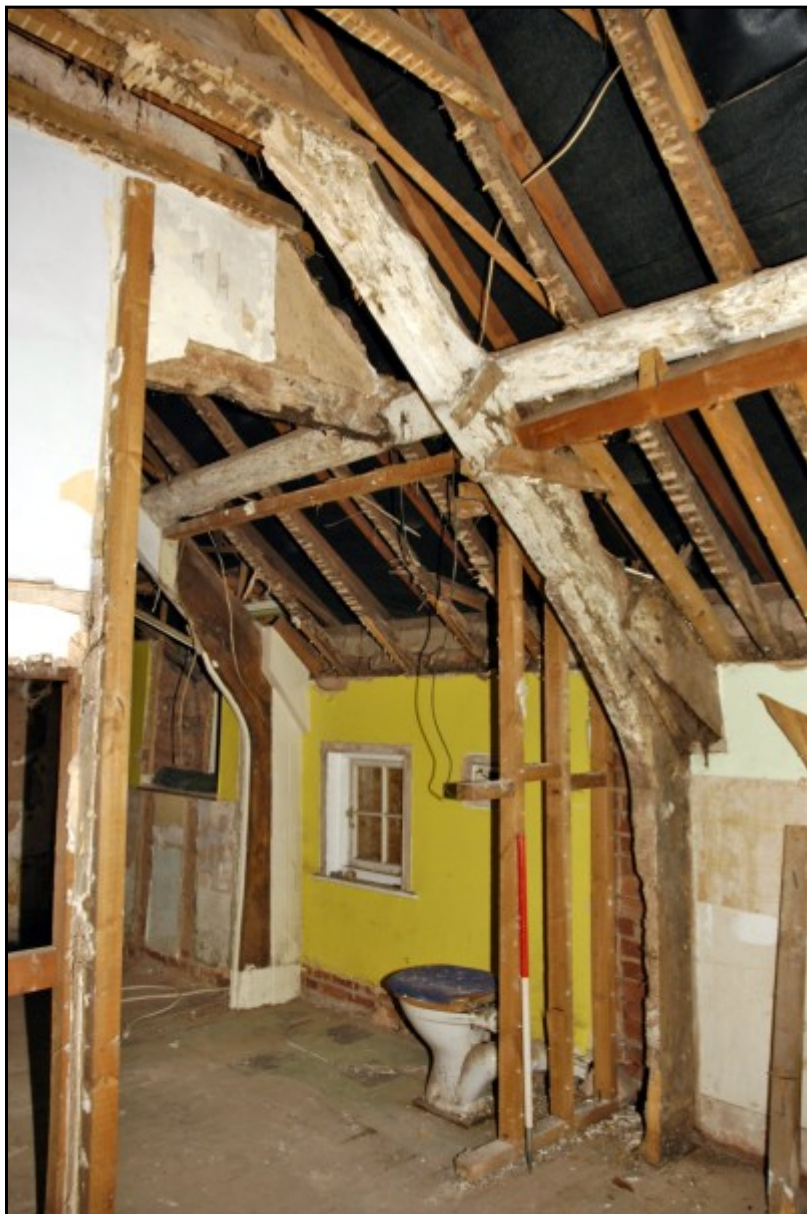
Fig. 17 Detail of the roof construction at the rear of the building showing two of the primary trusses and the rebuilt rear wall.
