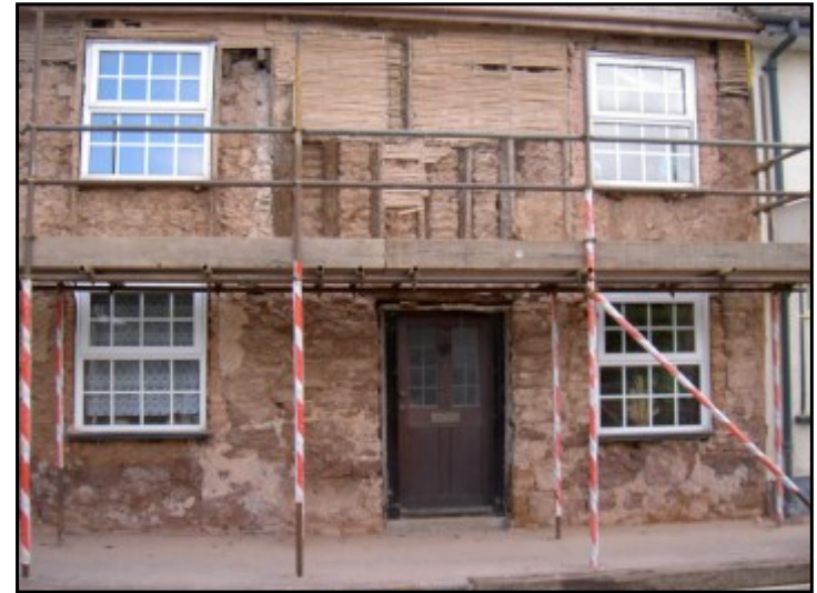
Fig. 5 Detail of the front of the cottage following the removal of the render in 2004, showing features in the southern part of the front wall (A. R. Pye, 2004).
