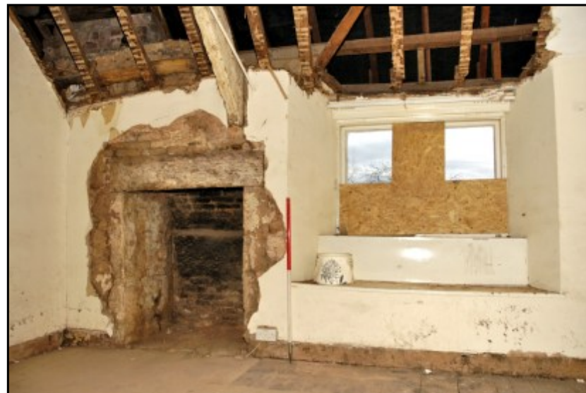
Fig. 18 View of the first-floor fireplace, window and roof truss in the front wall at the southern end of the inn.
