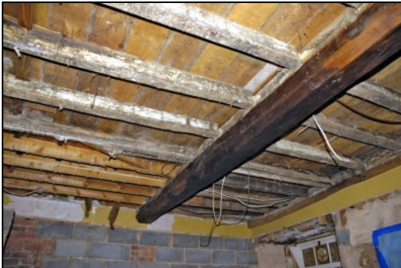
Fig. 11 View of the ceiling following stripping showing primary joists and the probable position of an inserted staircase infilled with modern joists (bottom left).
