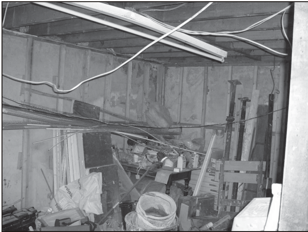
Fig. 8 The rear room, ground floor at the time of recording, showing party wall (left), back of chimney breast, and modern joists.
