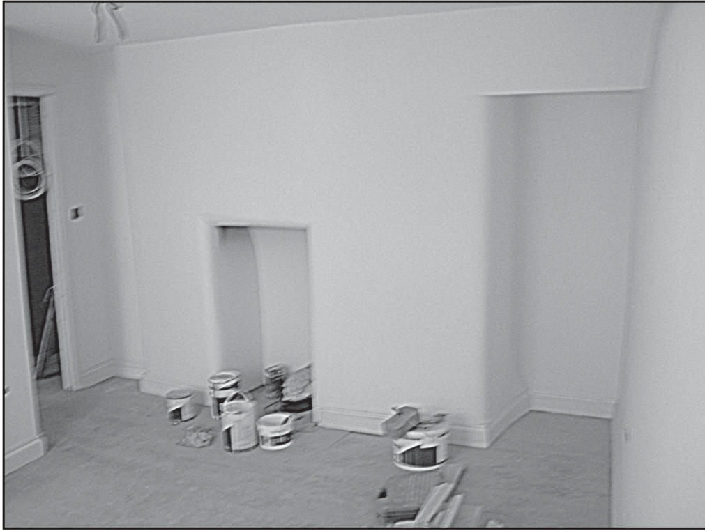
Fig. 12 Front room, first floor at the time of recording, showing 17C fireplace (left), and later doorway cut through adjacent wall (right).
