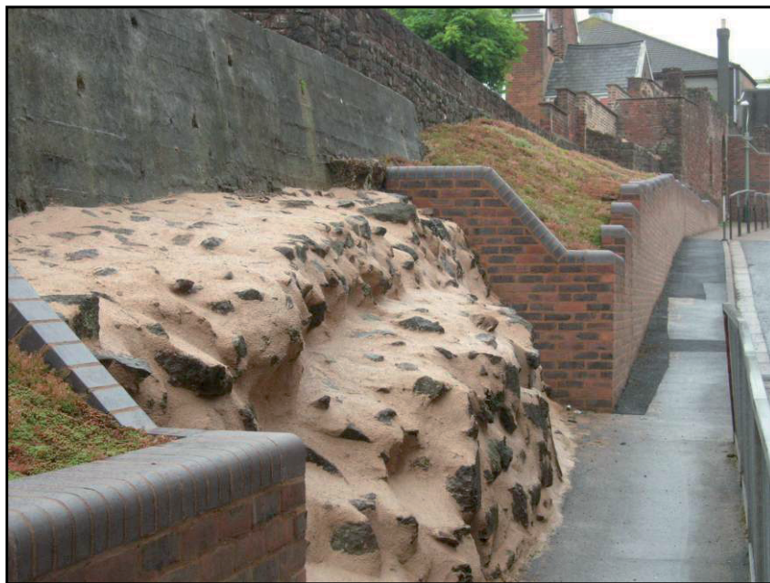
Plate 2. General view of site after completion of retaining wall and consolidation work, looking NE.
