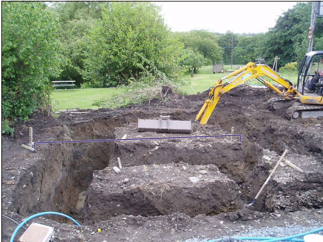
Pl. 1 Working shot looking northeast. The clayey fills of feature 104 can be seen in the deep foundation trench to the left. Blue line indicates location of Section 1.
