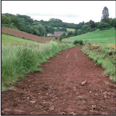
Plate 1 Pipeline route after turf removal. View to south-east, showing Haccombe House in background.
