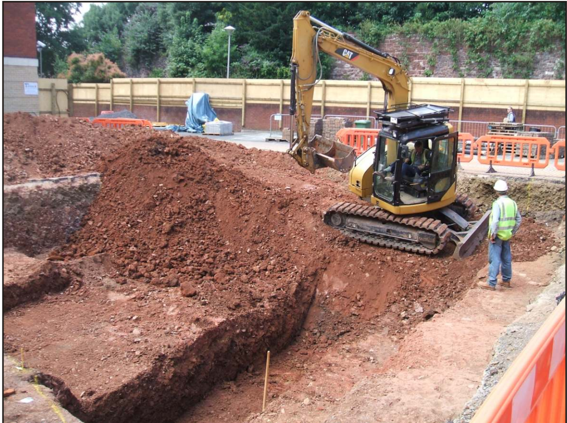
Plate 1 General view of site with hotel to left and city wall in background. View to west.
