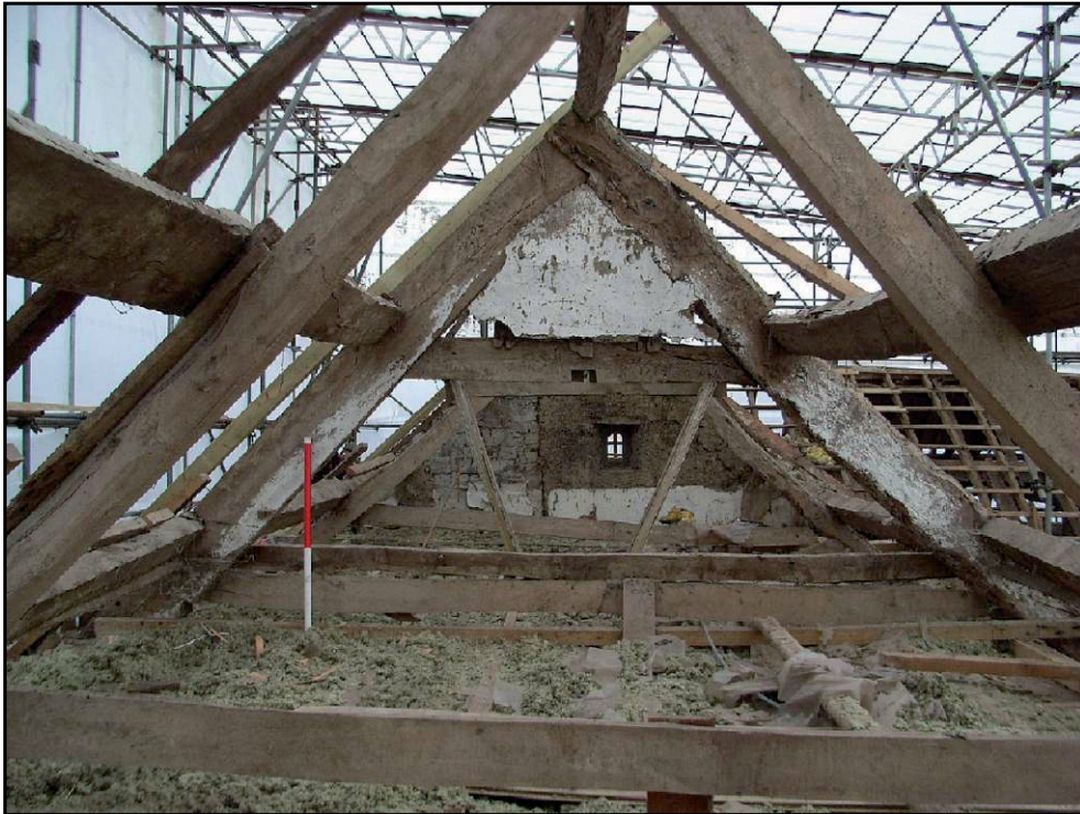
Pl. 1 The eastern principal truss in the north range, looking east. 1m scale.
