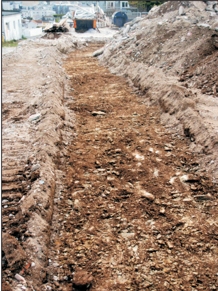
Plate 3 General view of trench showing natural subsoil immediately below sub-base. Looking east.
