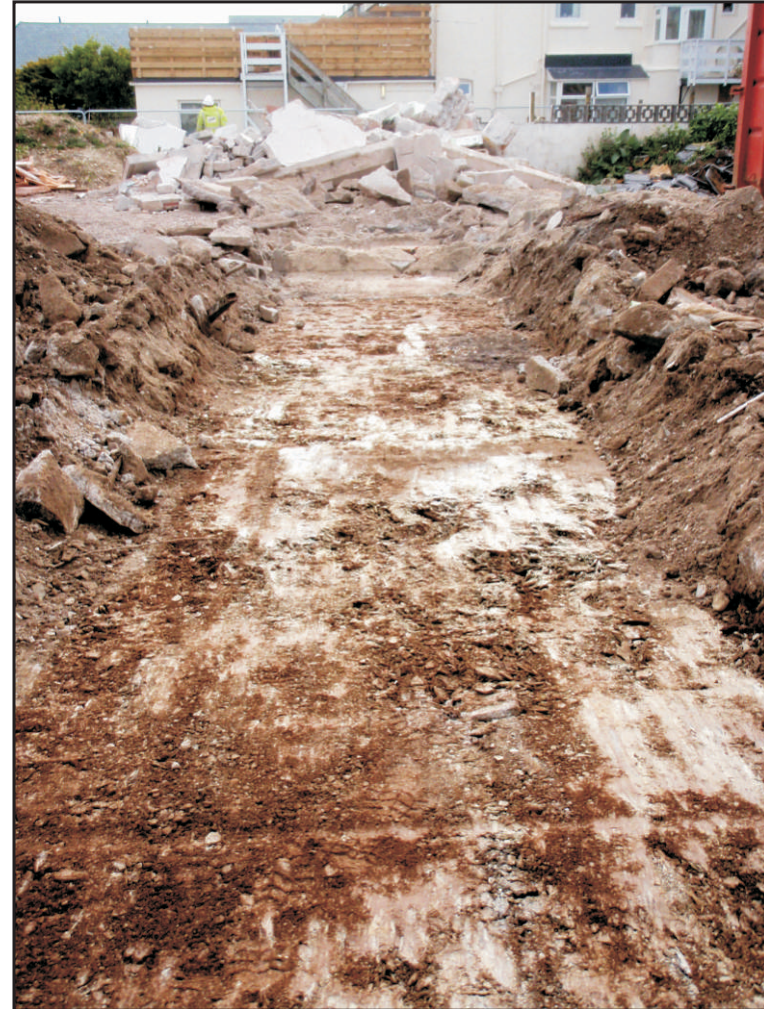
Plate 4 General view of trench showing natural subsoil immediately below sub-base. Looking east.
