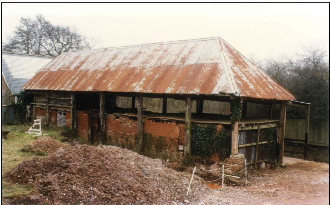
Fig. 17 View of the 17th- or 18th-century open-sided barn or linhay at Pinbrook House, Pinhoe, near Exeter, photographed in 1996. Included for comparison with the southern part of the building under discussion.
