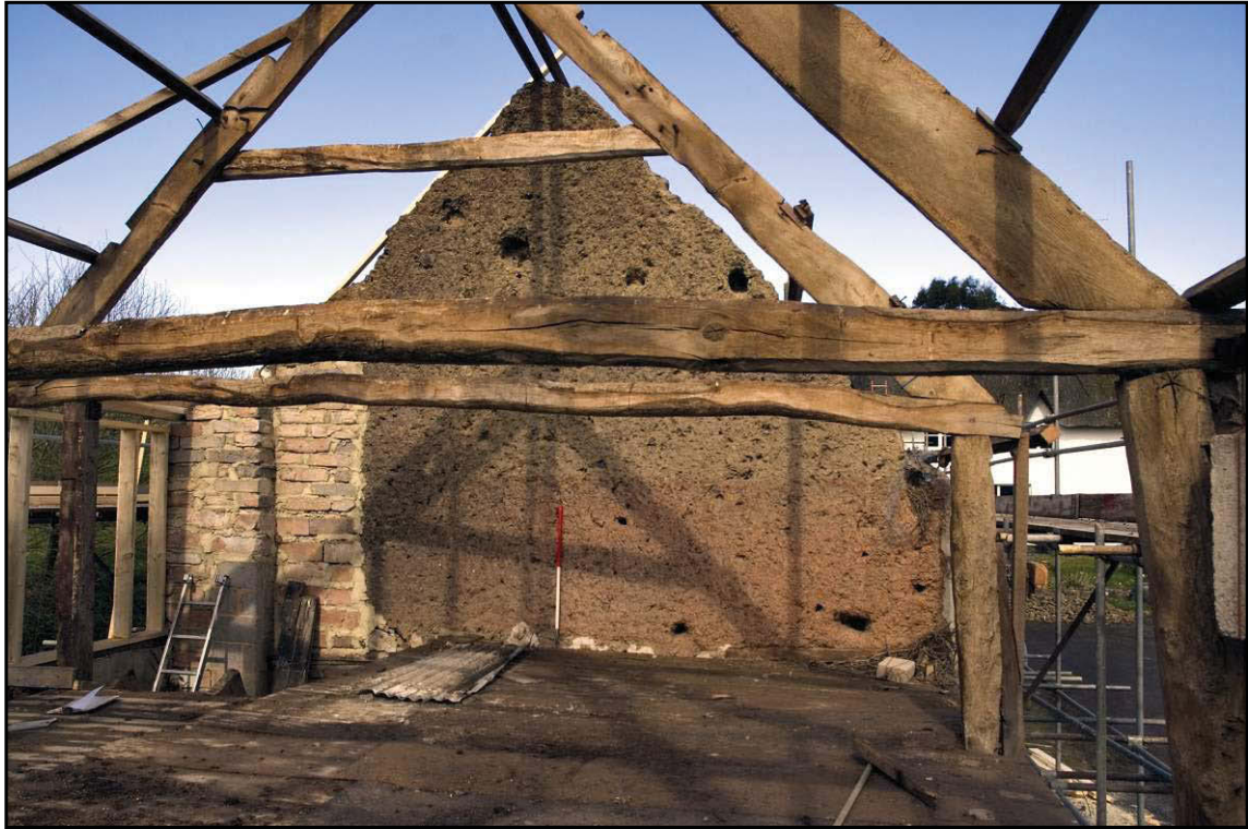
Fig. 6 View of the upper floor of the linhay showing the roof construction and the cob wall with areas of modern patching between the linhay and the barn.
