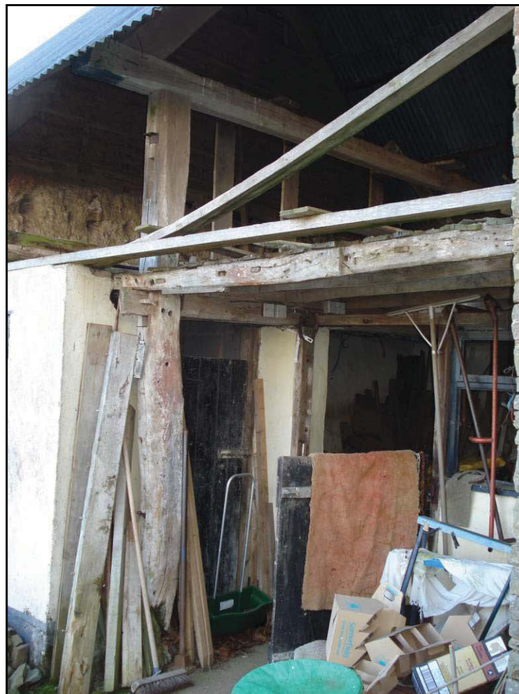
Fig. 13 Detail of the construction of the linhay to the north of the barn showing the post resting on a staddle, the projecting tenon at first-floor level and the mortice betraying the former high level of the floor.
