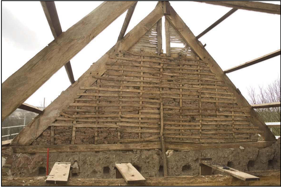
Fig. 12 View of the timber-framed partition at the north end of the barn showing the cob infill held in position by cleft laths and the ventilator at the apex.
