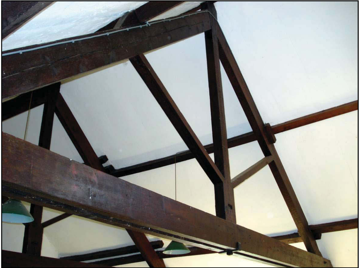
Fig. 16 Detail of the replacement roof trusses over the northern end of the building.
