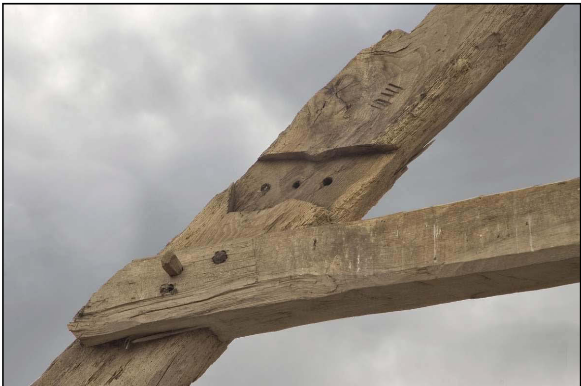
Fig. 7 Detail of one of the roof trusses showing carpenters' marks, redundant sockets for the collars and for trenched purlins and the fixings of the applied collars.
