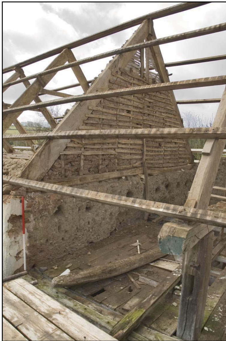
Fig. 14 View at first-floor level showing the sockets for the raised floor level in the linhay north of the barn and its relation to the roof structure.
