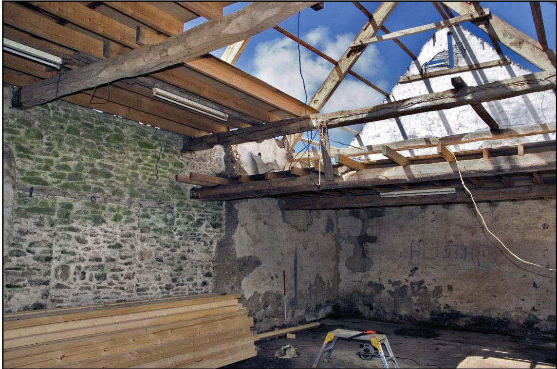
Fig. 10. View of the interior of the barn showing the character of the roof, the plastered walls and the blocked openings and stone intrusions in the west wall.
