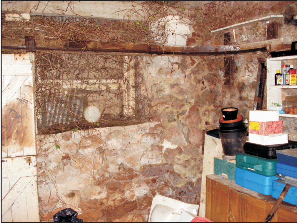
Fig. 9 Detail of the interior of the east wall showing the possible early fabric below the window.
