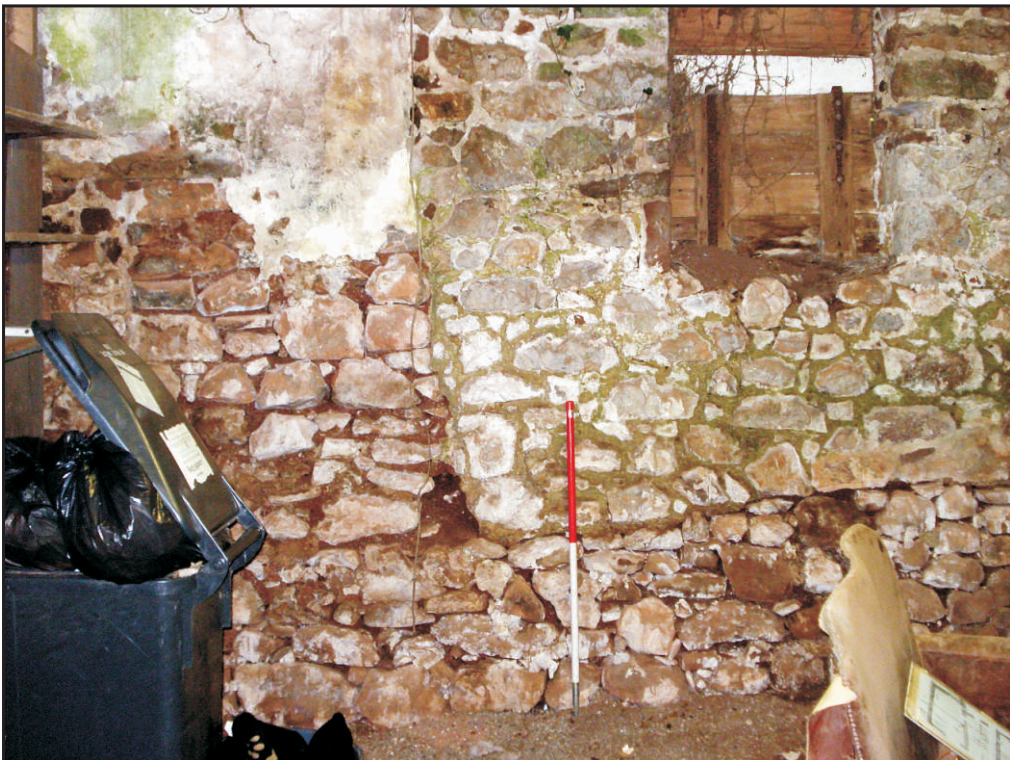
Fig. 10 Internal view of the south wall showing building breaks and features in the western part of the structure.
