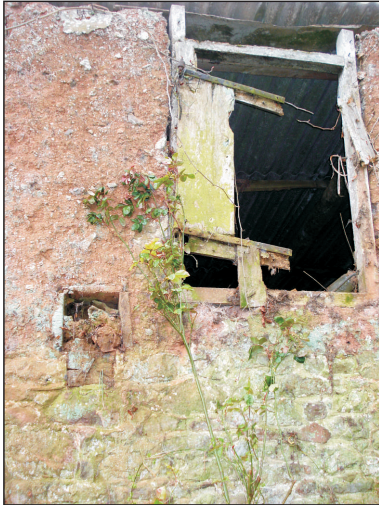
Fig.4 Detail of the first-floor loading door in the north elevation showing the reinforced socket below the doorway.
