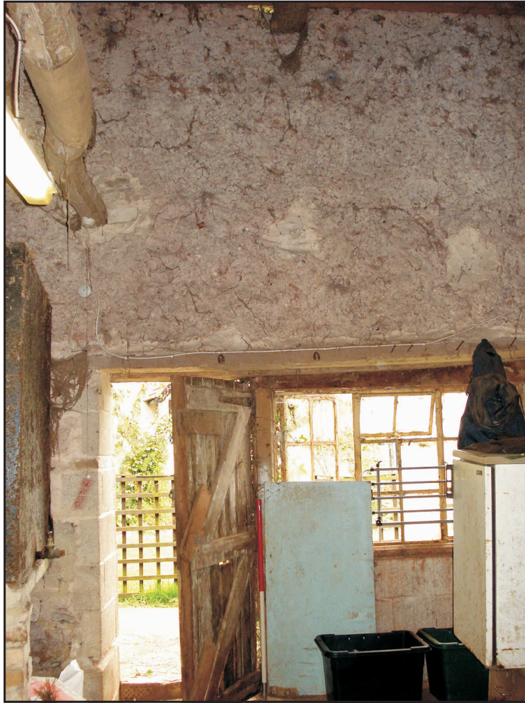
Fig. 8 Internal view of part of the north wall showing the sockets for vanished beams.
