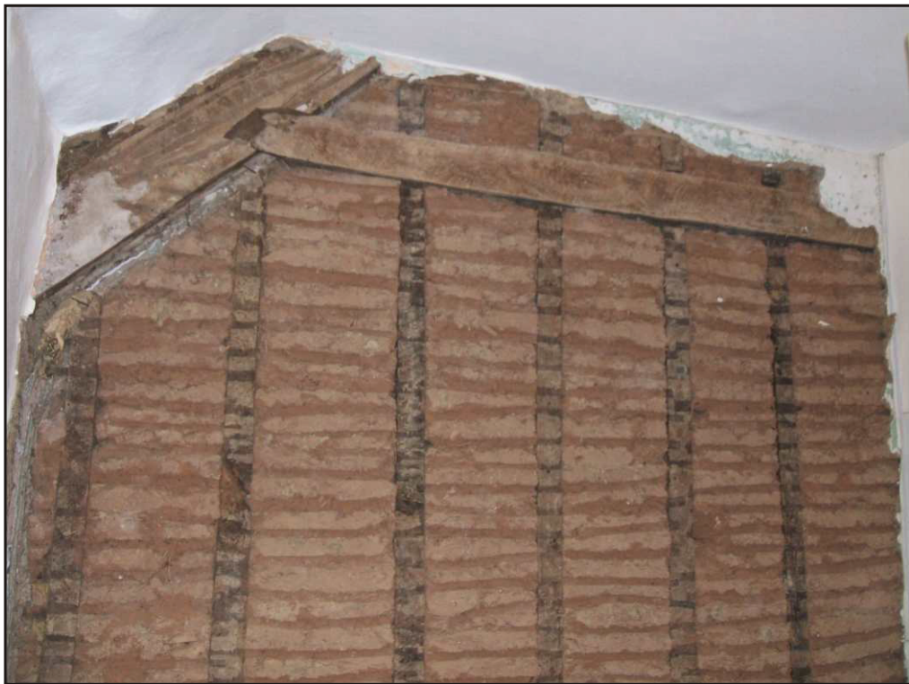
Plate 2 The western partition showing the collar and partition dropping from the truss, looking west.
