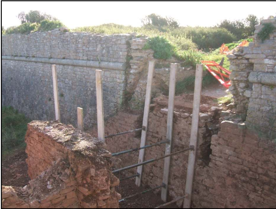
Pl. 1 Fort 1: entrance showing pier, and chases for timbers on the curtain wall, looking south-east.
