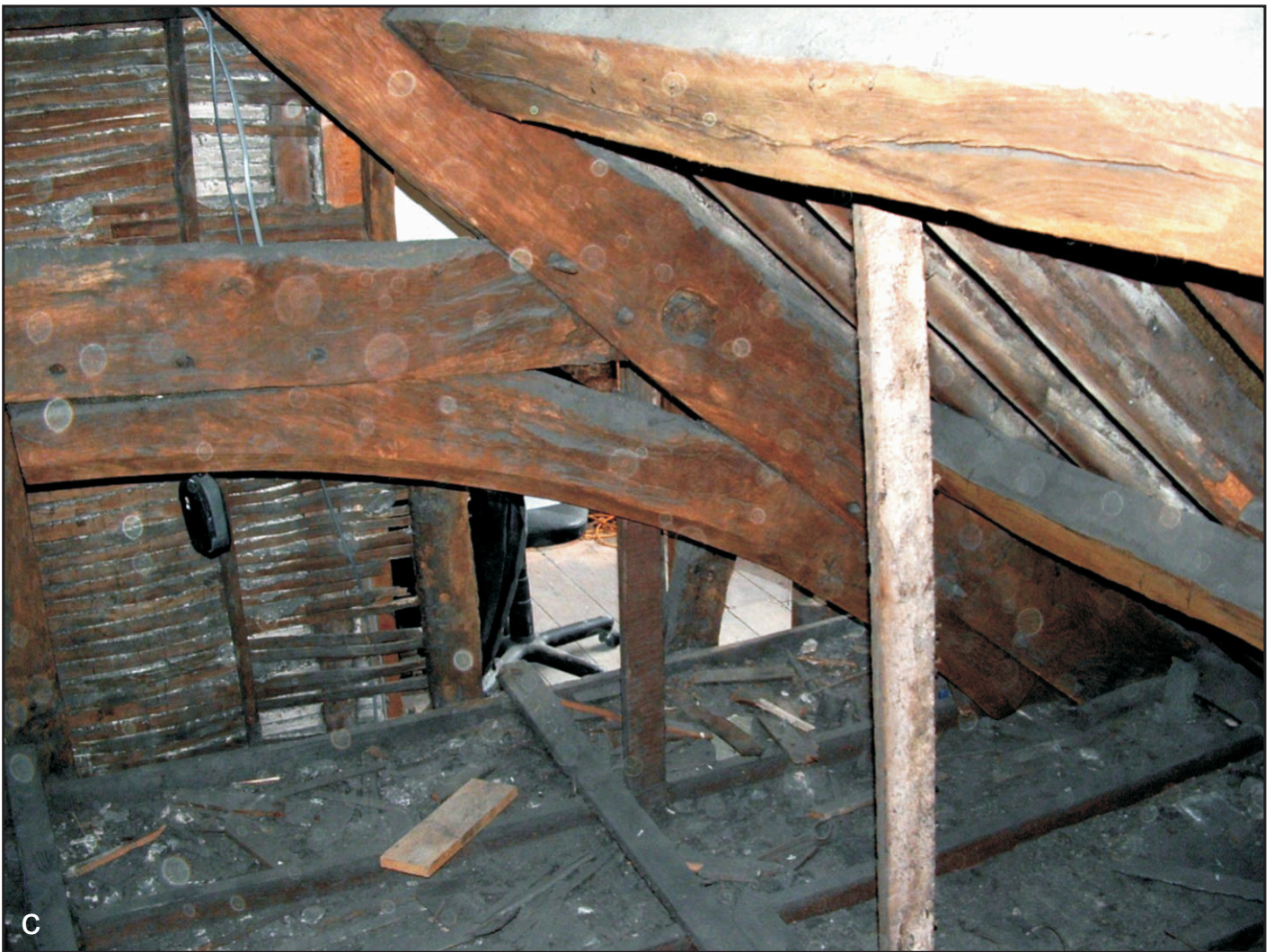
Fig. 4a-c Roof 1, Truss 2 with 17th-century partition beyond, from SW.
