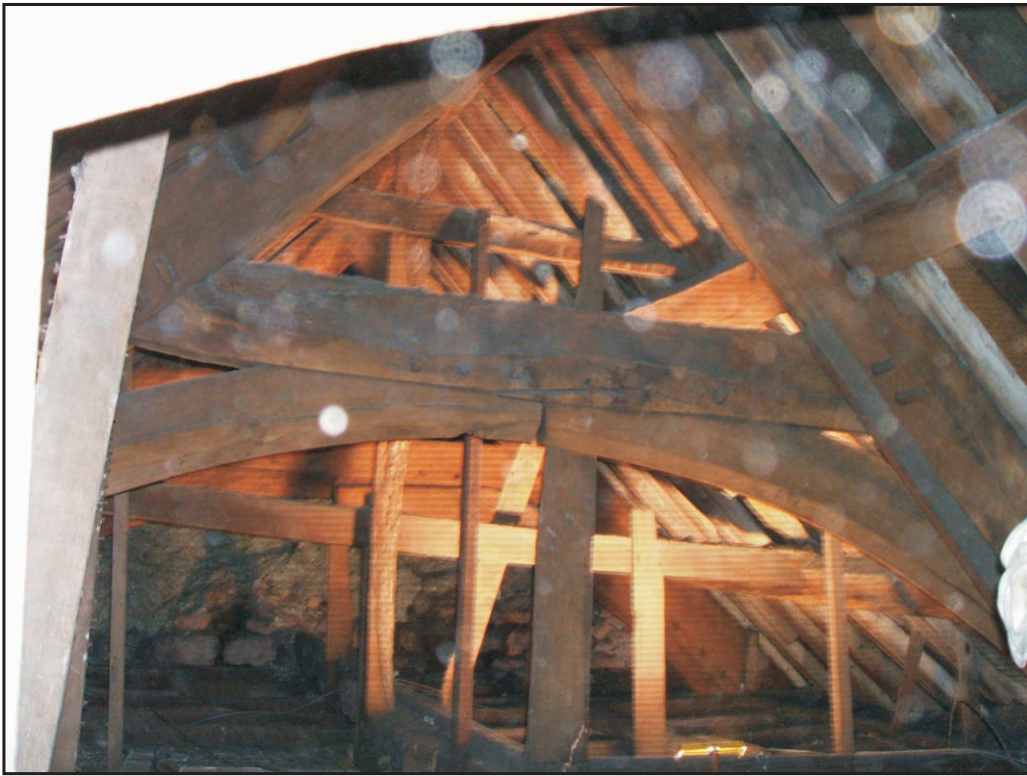
Fig. 3a Roof 1 looking SW, with Truss 3 in the foreground and the wall-top of the front range visible below insulating material in the background.
