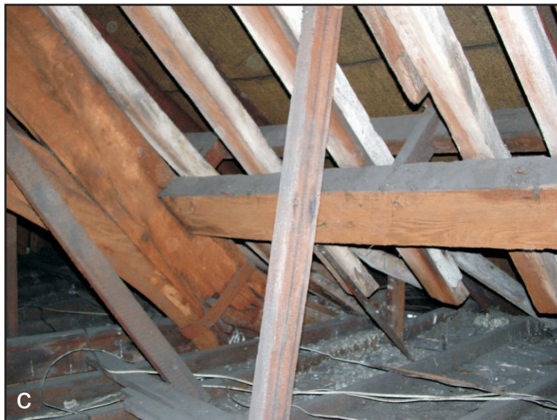
Fig. 5a-c Roof 1, Truss 3 from the NE and NW, the latter showing later strapping of the principal.
