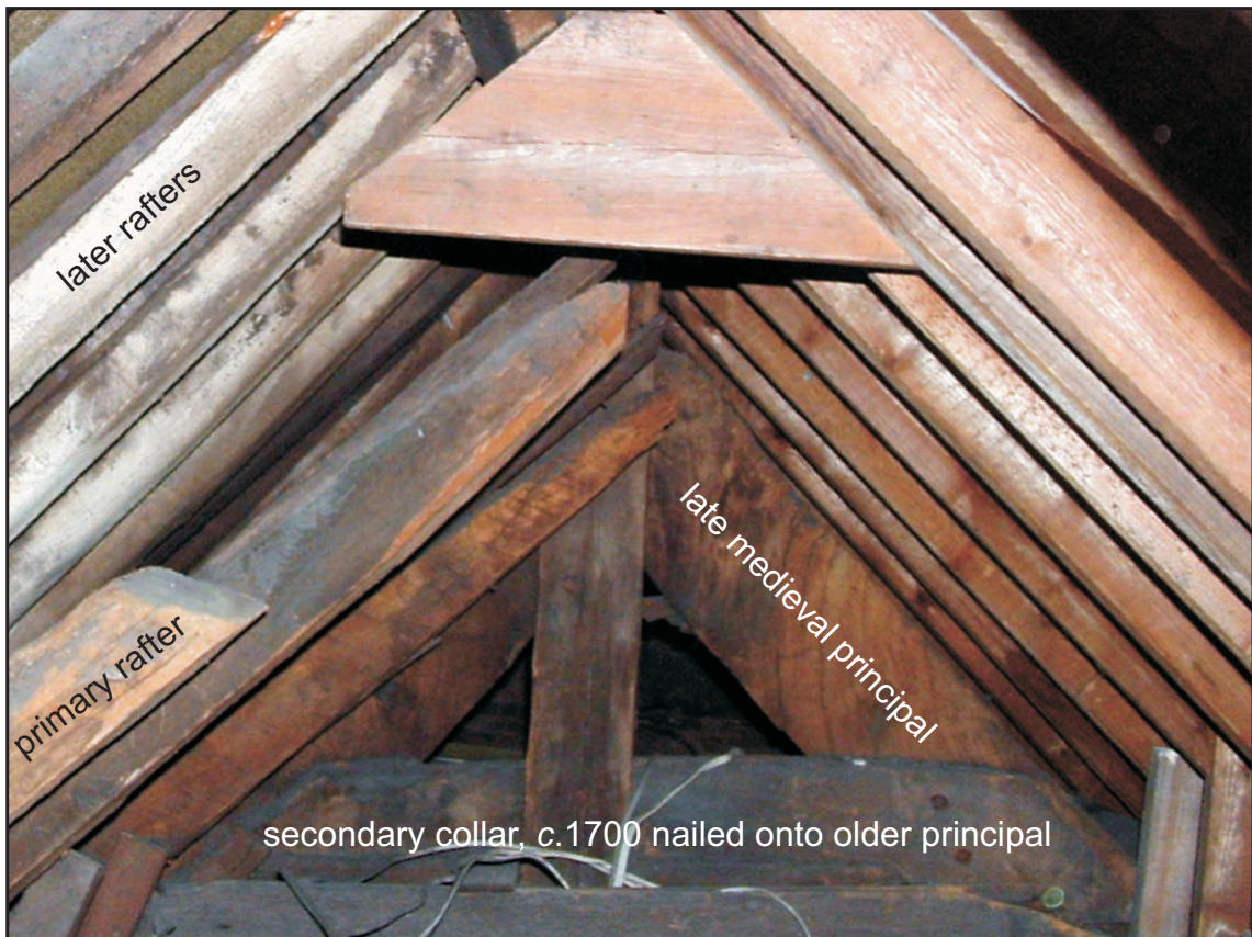
Fig. 8b The top of Roof 2, seen in the roofspace above its ceiling.
