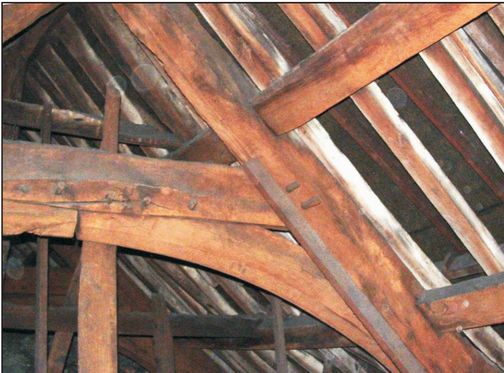
Fig. 3b Roof 1, Truss 3 from the NE, showing upper and middle purlins and arch bracing.
