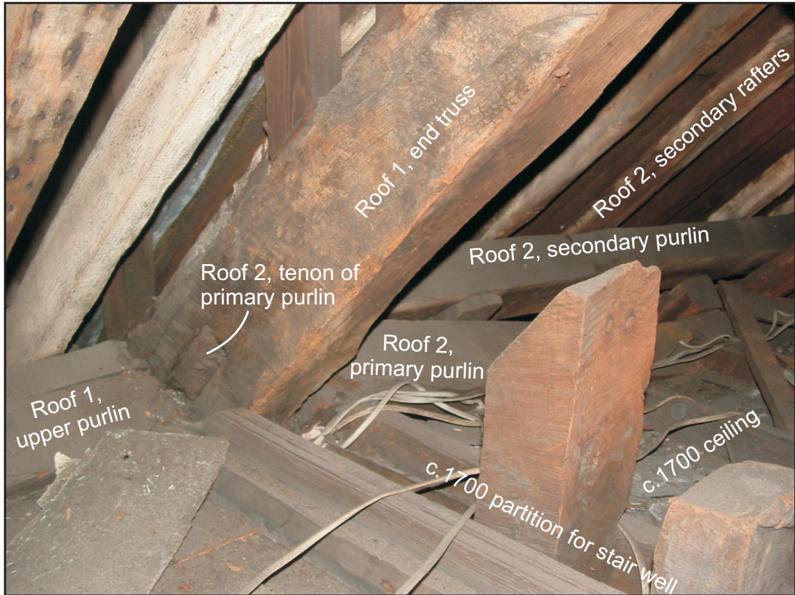
Fig. 8a The top of Truss 1 from the SW, showing principal and purlin of Roof 1, inserted tenon for purlin of Roof 2, distorted purlin of Roof 2 and later replacement roof-slope of Roof 2. The vertical timbers at the front are the top of the 17th-century studs added into Truss 1.
