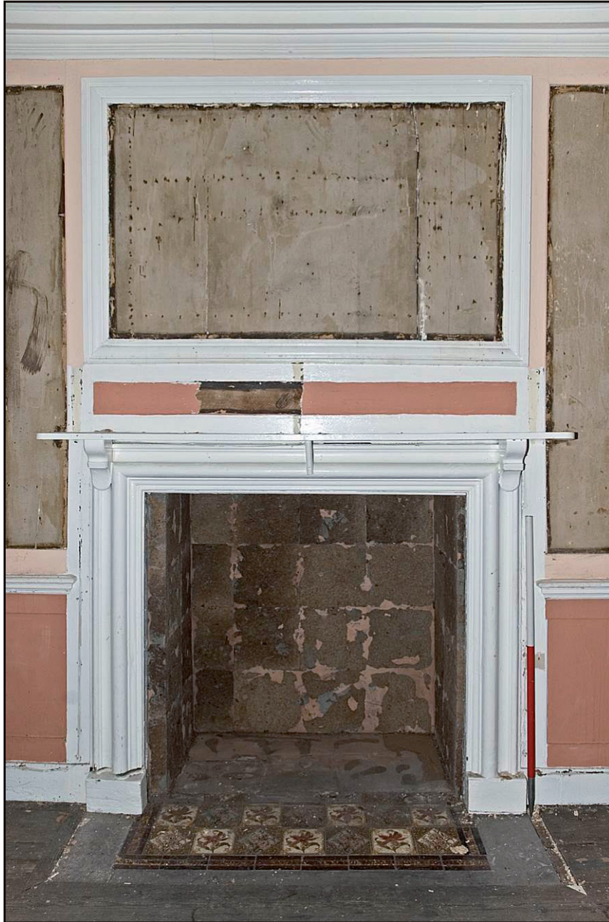
Fig. 14 View of the fireplace in the first floor, south-east room, showing the pattern of nail marks. Scale 1m. View south.
