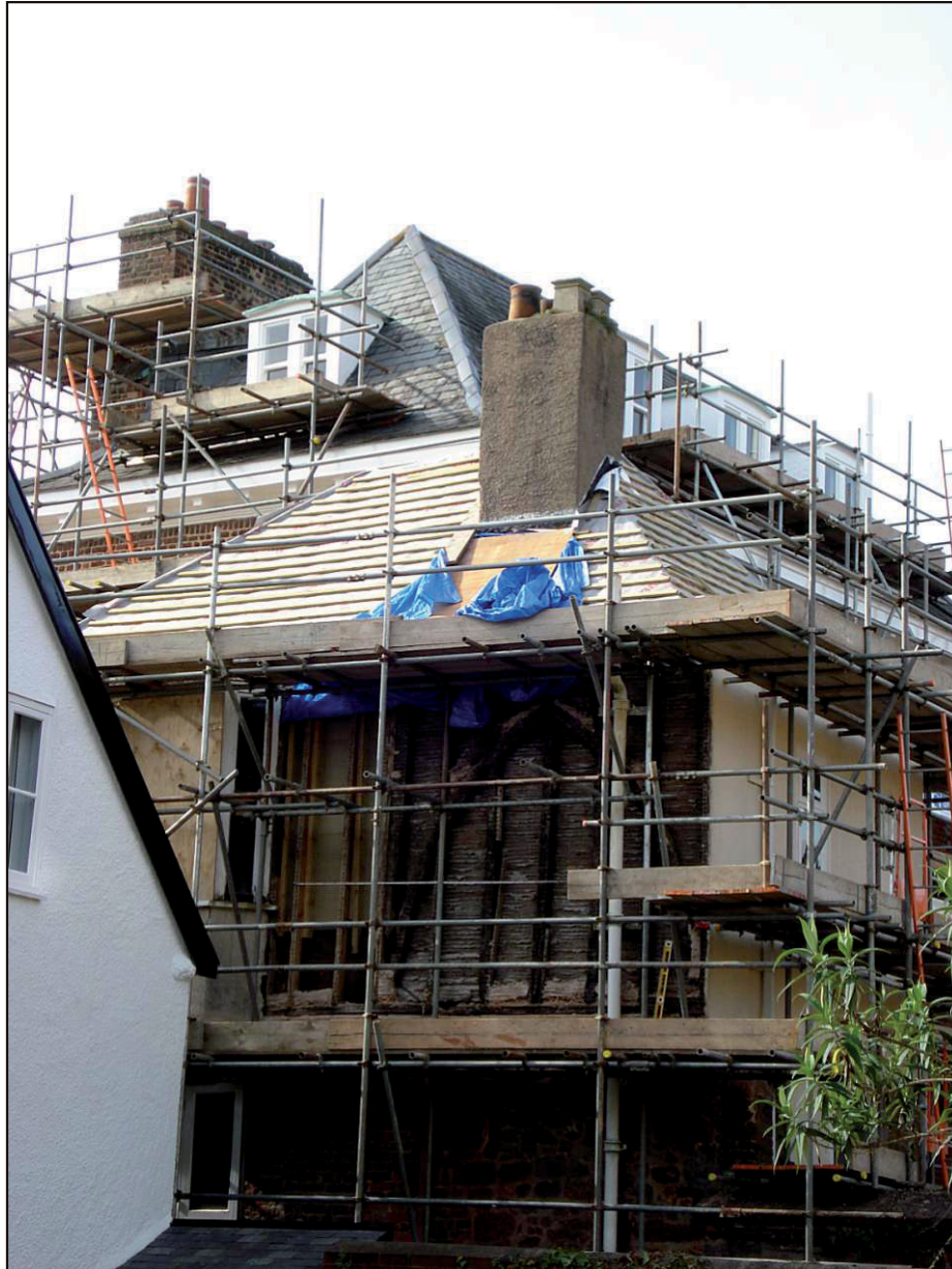
Fig. 3 View of the pavilion block showing the exposed framing prior to repairs.
