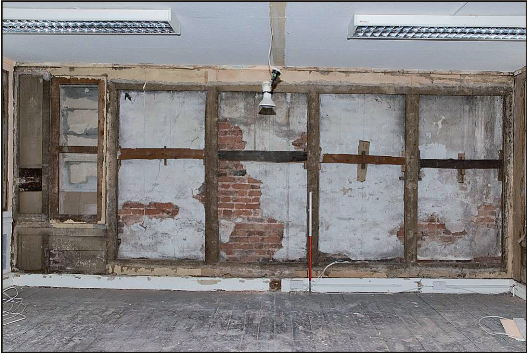
Fig. 17 View of the panelling on the south-eastern wall of the second floor south-east room. Scale 1m. View east.
