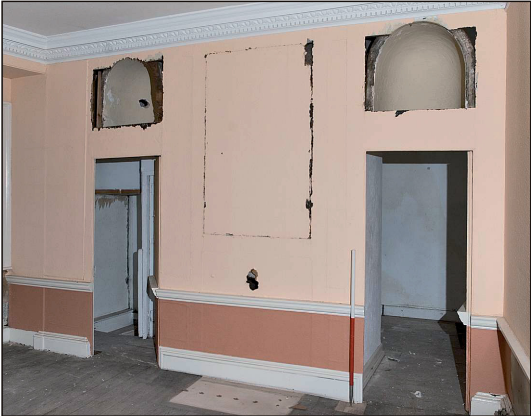
Fig. 15 View of the screen in the pavilion block showing the niches. Scale 1m. View north-west.
