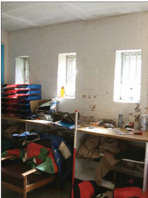
Plate 3 The interior of the Report and Control Centre showing barred windows and scars of removed partitions, looking east. 1m scale.
