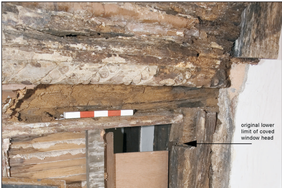
Pl. 16 Detail of the east end of the first-floor covered window head showing the lowest extremity of the beam surviving truncation for later windows (arrowed). Scale 0.25m. View south.
