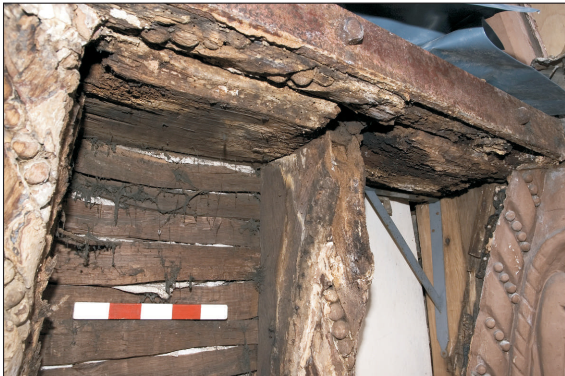
Pl. 4 Second-floor windowsill beam with spiral ribbon and bead moulding clamped between steel straps. Modern panel infills have been removed from between the jetty brackets. Scale 0.25m. View south.
