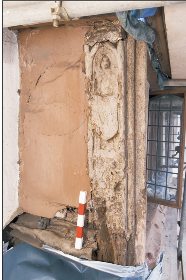
Pl. 9 View of the second-floor corner post at the east end showing lancet and shield carvings after limited paint stripping. Scale 0.25m. View south-west.
