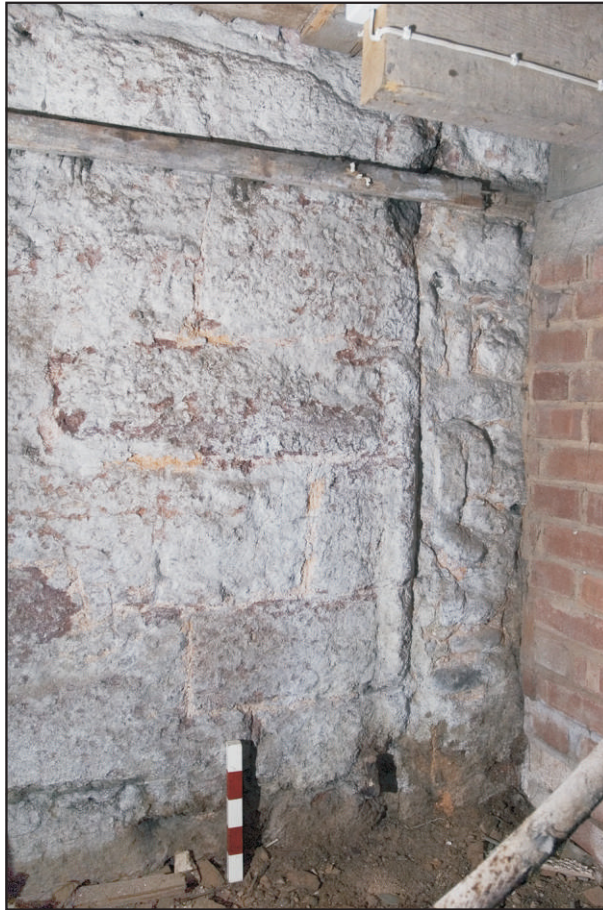
Pl. 18 View of the south-west cellar wall showing a blocked doorway with a rolled edge to the jamb and an iron pintle below. Scale 0.25m. View south-west.
