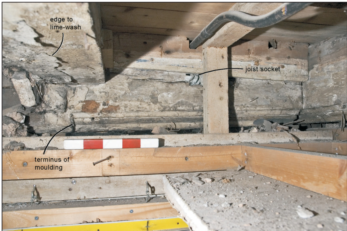
Pl. 24 View of the short section of moulded beam in the ground-floor ceiling of the north-west room overlying the site of the former passage. Note how the terminus of the moulding is aligned with a straight edge to limewash on the adjoining joist. Scale 0.25m. View north-west.
