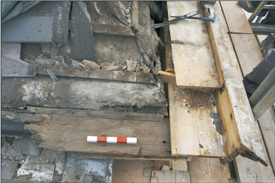
Pl. 20 View of the north-east corner of the roof showing the remnant of a timber base to a former parapet gutter that was later made redundant following the in-fill of Lamb Alley with No. 45. Scale 0.25m. View south-west.
