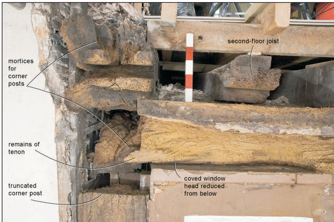
Pl. 15 Detail of the east end of the second-floor covered window head showing the remains of joints to adjacent timbers and the resulting gap created by truncation of the head beam following the insertion of later windows. Scale 0.25m. View south-east.
