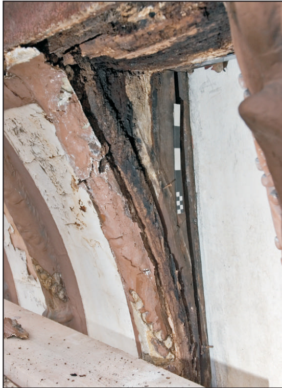
Pl. 5 Detail of a second-floor covered jetty bracket after removal of the modern panel showing the grooves for lath and plaster infill. Scale 0.25m. View east.
