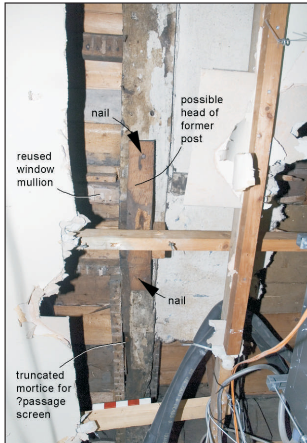
Pl. 22 View of the ground-floor ceiling of the north-west room showing the joist with a truncated mortice for a possible passage screen and the remains of a possibly later post. Scale 0.25m. View south-east.
