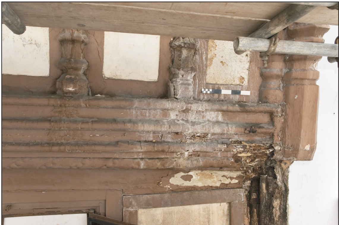
Pl. 6 Detail of the west end of the facade showing the deterioration of the timbers of the second floor. Scale 0.25m. View south-east.
