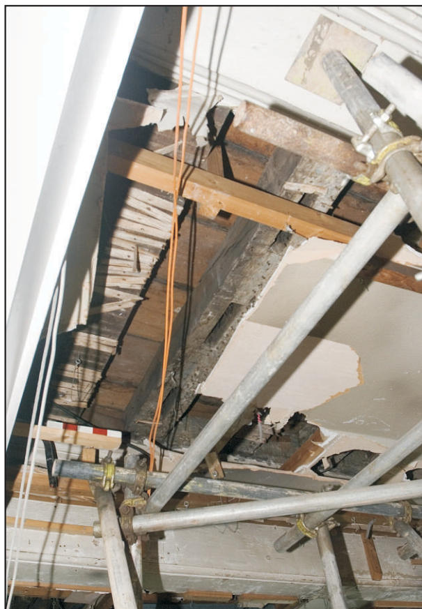
Pl. 21 View of the partially stripped ground-floor ceiling of the north-west room showing the joist with mortices for a former passage screen along the north-east side. Scale 0.25m. View south-east.
