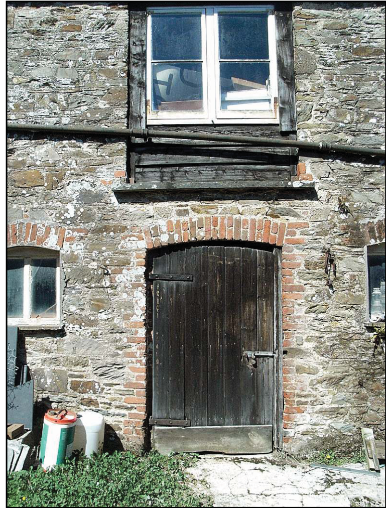
Plate 4 The stable door showing inconsistency in the brick dressings.
