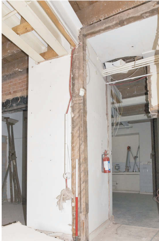
Photo 5. Original studwork between the front and rear rooms of the basement on the south-east side, with mortices for a stud and a possible door-head beam. Scale 1m. View north.
