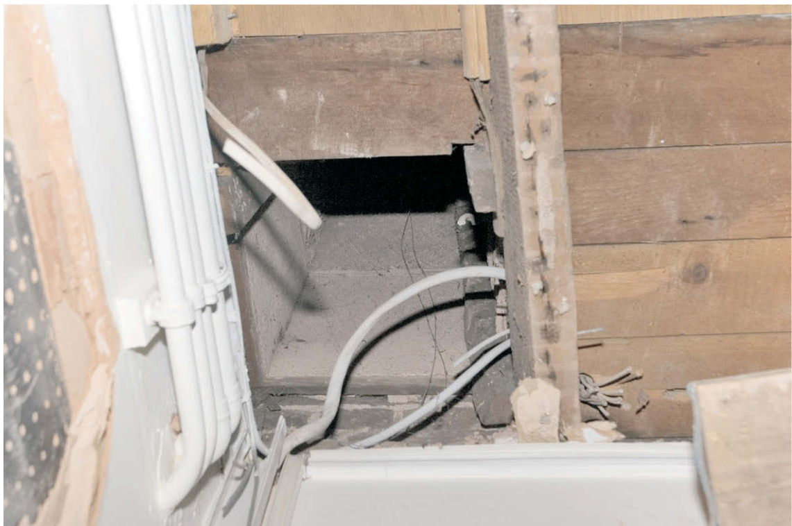
Photo 2. View of the possible service lift as seen from the basement rear room on the north-west side. View north-west.
