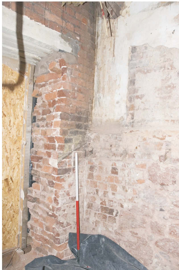
Photo 8. View of the original brickwork of the rear wall of the building at ground-floor level, showing the inserted door, with a concrete lintel, in the north-west corner. Scale 1m. View west.
