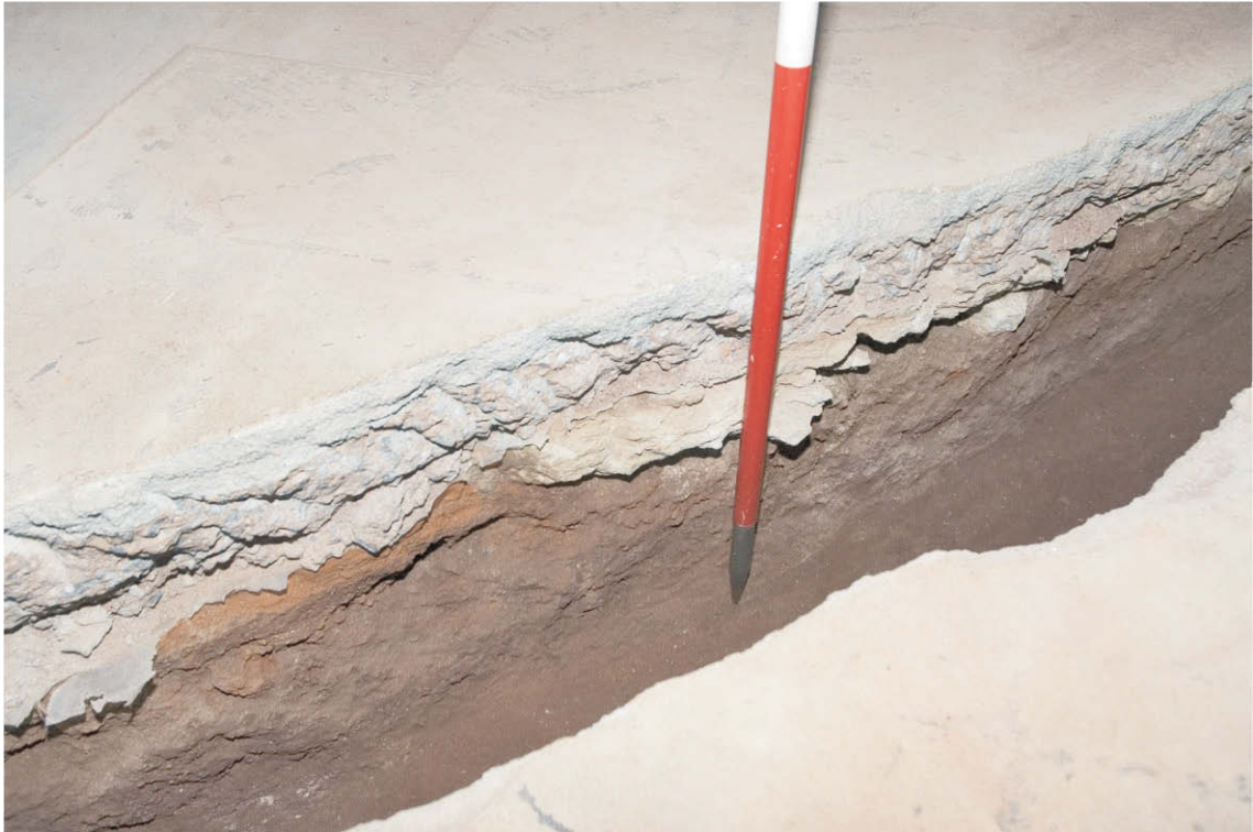
Photo 7. View of the drainage trench in the basement front room showing the southern limit of a flagstone floor below the modern concrete. Scale 1m (0.50m in view). View north-west.
