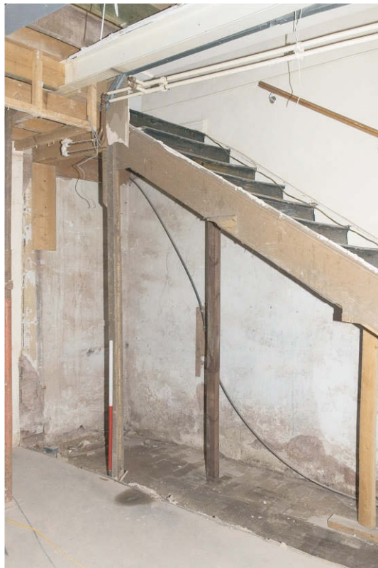
Photo 6. View towards the original basement stairs with an original brick floor below, exposed after the removal of a screen wall. Scale 1m. View east.
