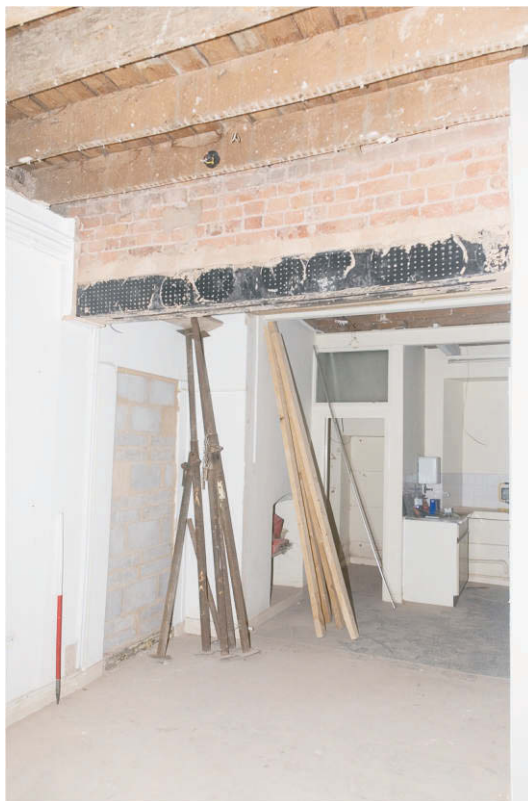
Photo 4. The front basement room showing the high-level remains of an original brick partition wall, supported by steelwork, that divided front from rear rooms on the north-west side. Scale 1m. View north.
